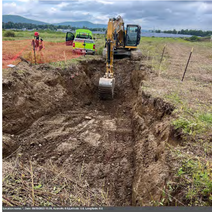
Photo 7: Excavation of buried receiver tube waste at south end of trench with silt fence
