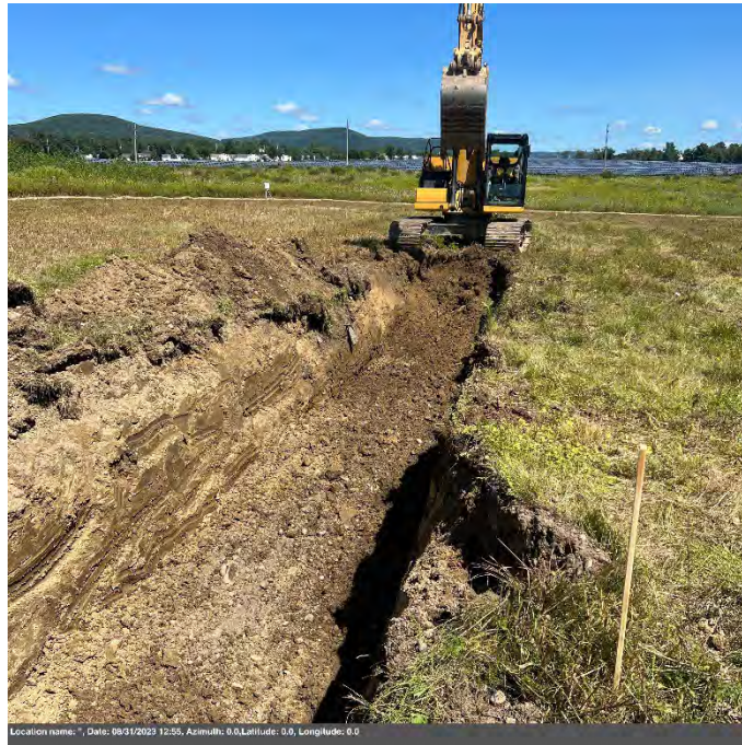
Photo 11: View facing north – excavation of receiver tube waste at north end of trench
