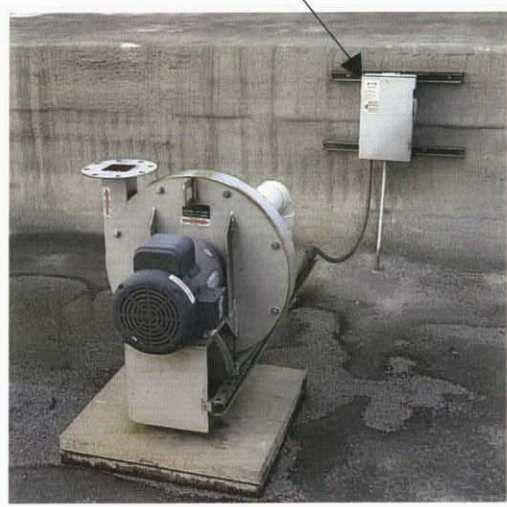
Building 25 Roof Mounted Fan
