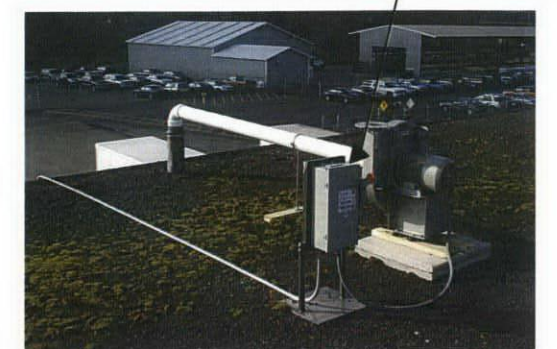
Buildings 8 and 15 Roof Fan
