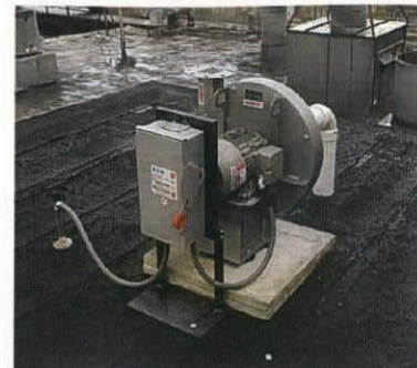
Buildings 11A-A, 11A-B, and 20 Roof Mounted Fan and Disconnect Switch
