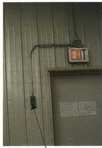
Disconnect Switch (located inside Bldg 31 on east wall beneath fan)
