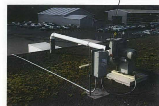
Buildings 8 and 15 Roof Fan
