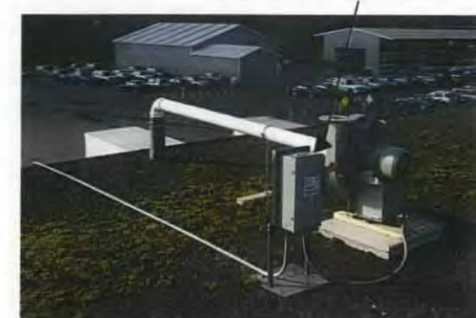
Buildings 8 and 15 Roof Fan
