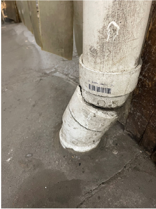
Photo 1 Broken riser pipe 20-4.
