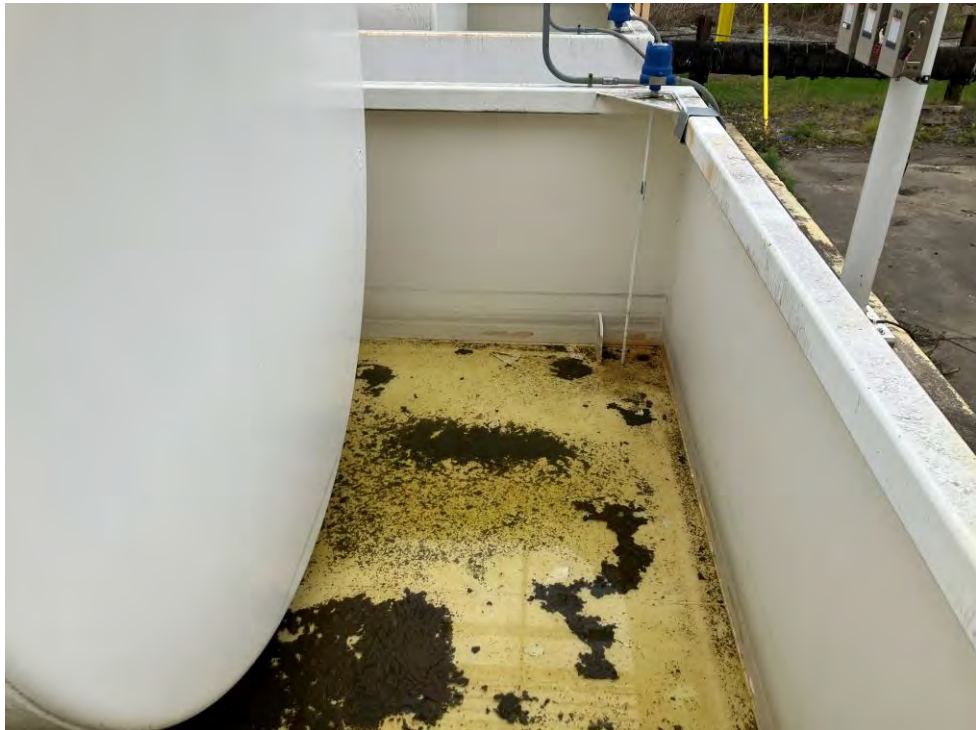
Photo 4 View of secondary containment associated with TBAC ASTs as they are being drained by Garlock personnel after the PRR reporting period.
