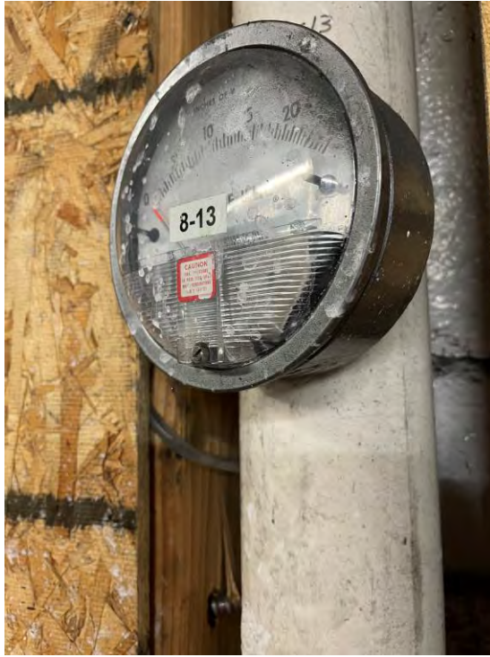
Photo 1 Magnehelic gauge 8-13 in Building 8 with tubing pinched behind sheathing.
