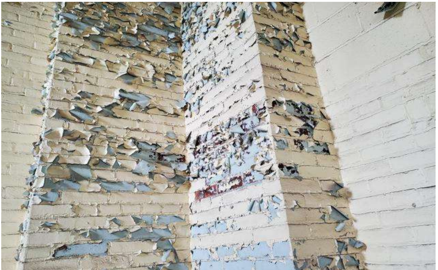
Suspected lead-based paint (LBP)
