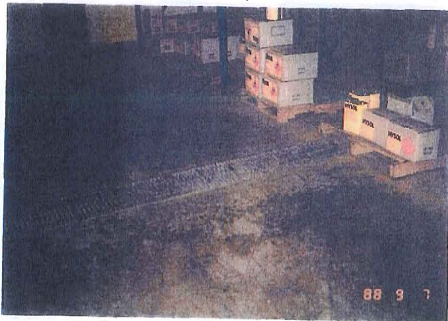
Date: 9/7/88 Picture Taken By: E. Lin Direction Facing: West Picture Description: The trough in the solvent storage room
