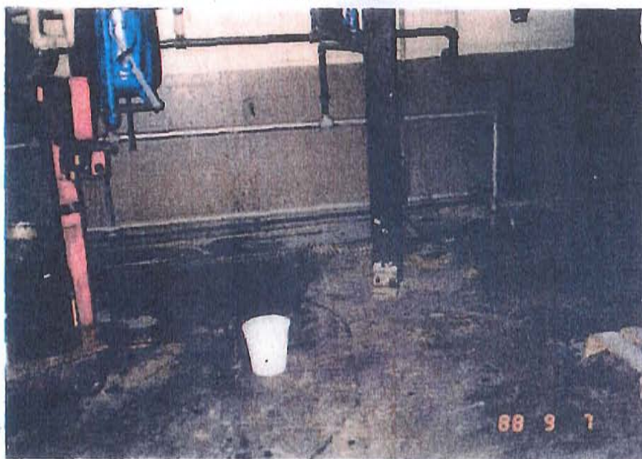
Date: 9/7/88 Picture Taken By: E. Lin Direction Facing: _____ Picture Description: The drain in the form solvent reclamation unit area.
