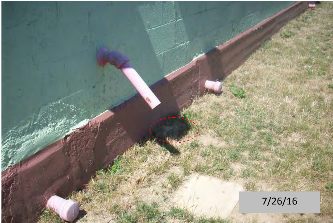
View of area where animal burrow was noted in the soil cover during 6/29/16 site-wide inspection, and was subsequently repaired with the addition of supplemental cover soil.
