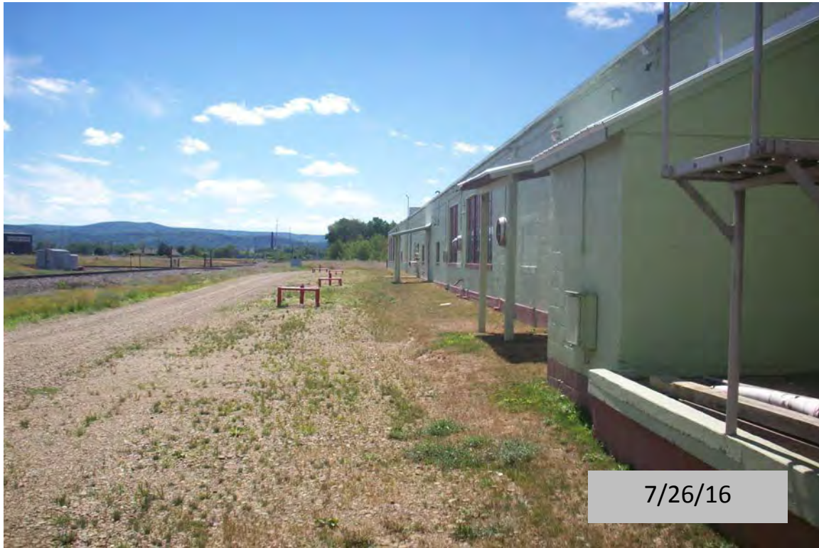
View, facing west, of the soil cover over the southern edge of the Site
