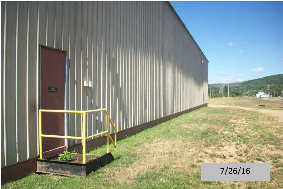
View, facing east, of the soil cover over the southern edge of the Site
