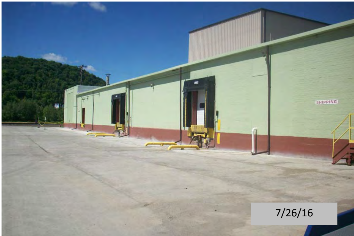
View, facing north, of the concrete pavement cover over the shipping lot on the west portion of the Site
