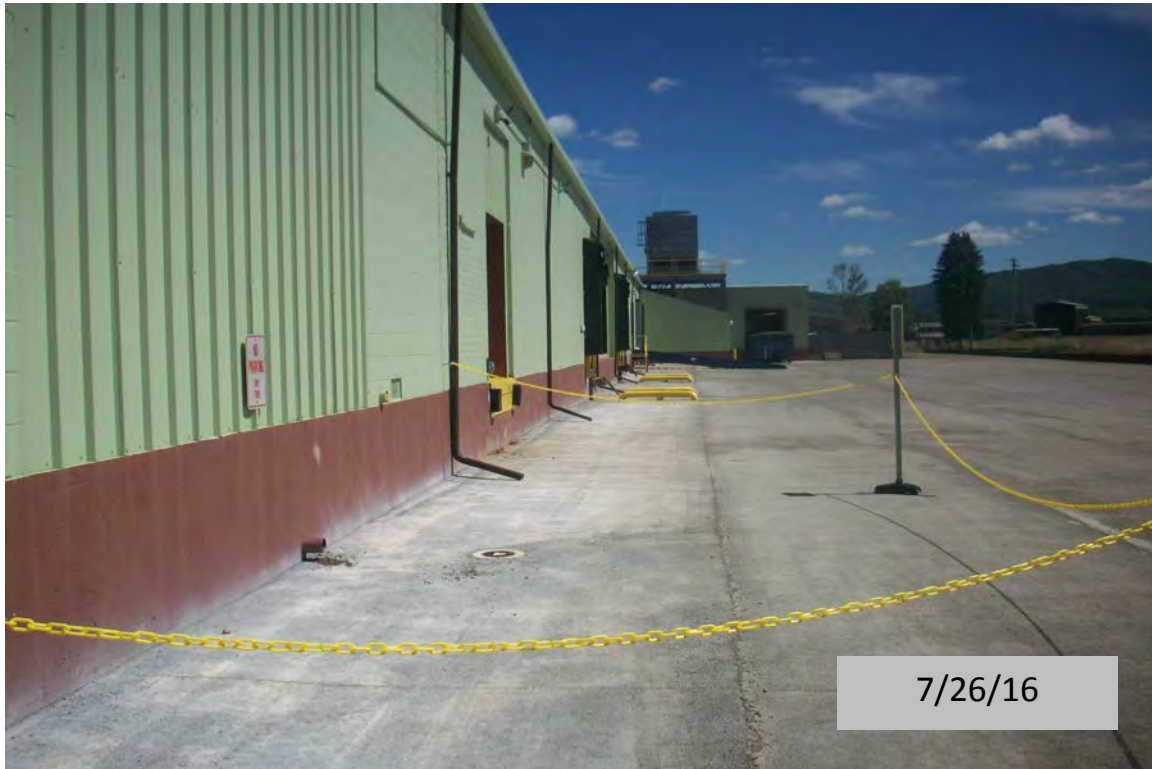
View, facing south, of the concrete pavement cover over the shipping lot on the west portion of the Site.
