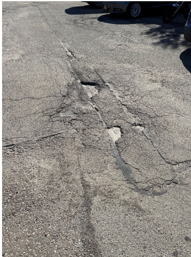
View of deteriorating asphalt pavement cover located in the south-central portion of the Employee Parking Lot, facing southeast
