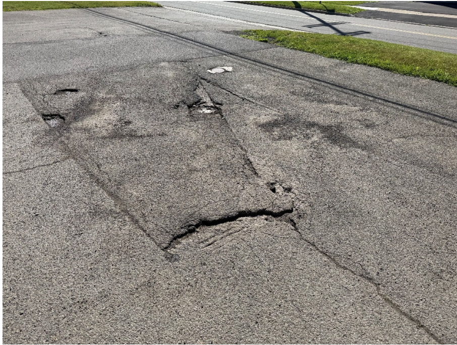
View of deteriorating asphalt pavement cover located in the southeast portion of the Employee Parking Lot, facing southeast
