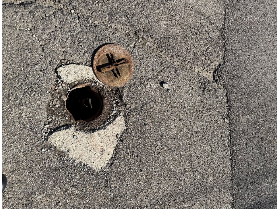
View of deteriorating concrete surface seal surrounding the curb box for MW-F, located in the southeast portion of the Employee Parking Lot.
