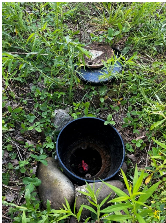
View of a flush-mounted monitoring well curb box MW-E and surrounding much cover located on the eastern portion of the Site.
