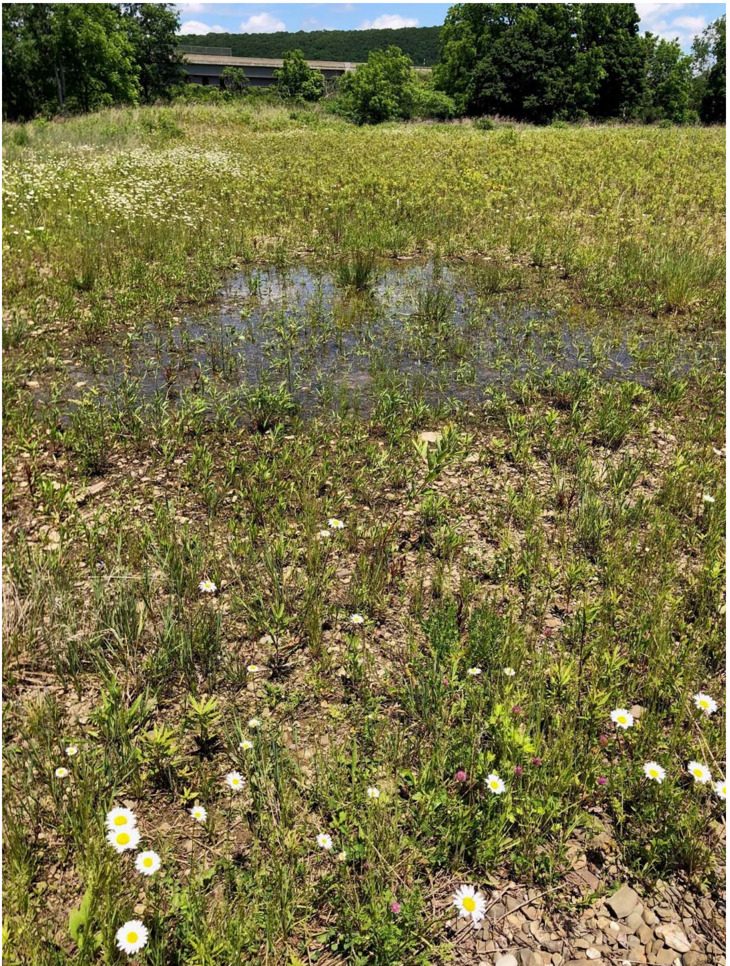
View of an area of standing water observed near the drainage channel, located on the northwest portion of the Site, facing north.
