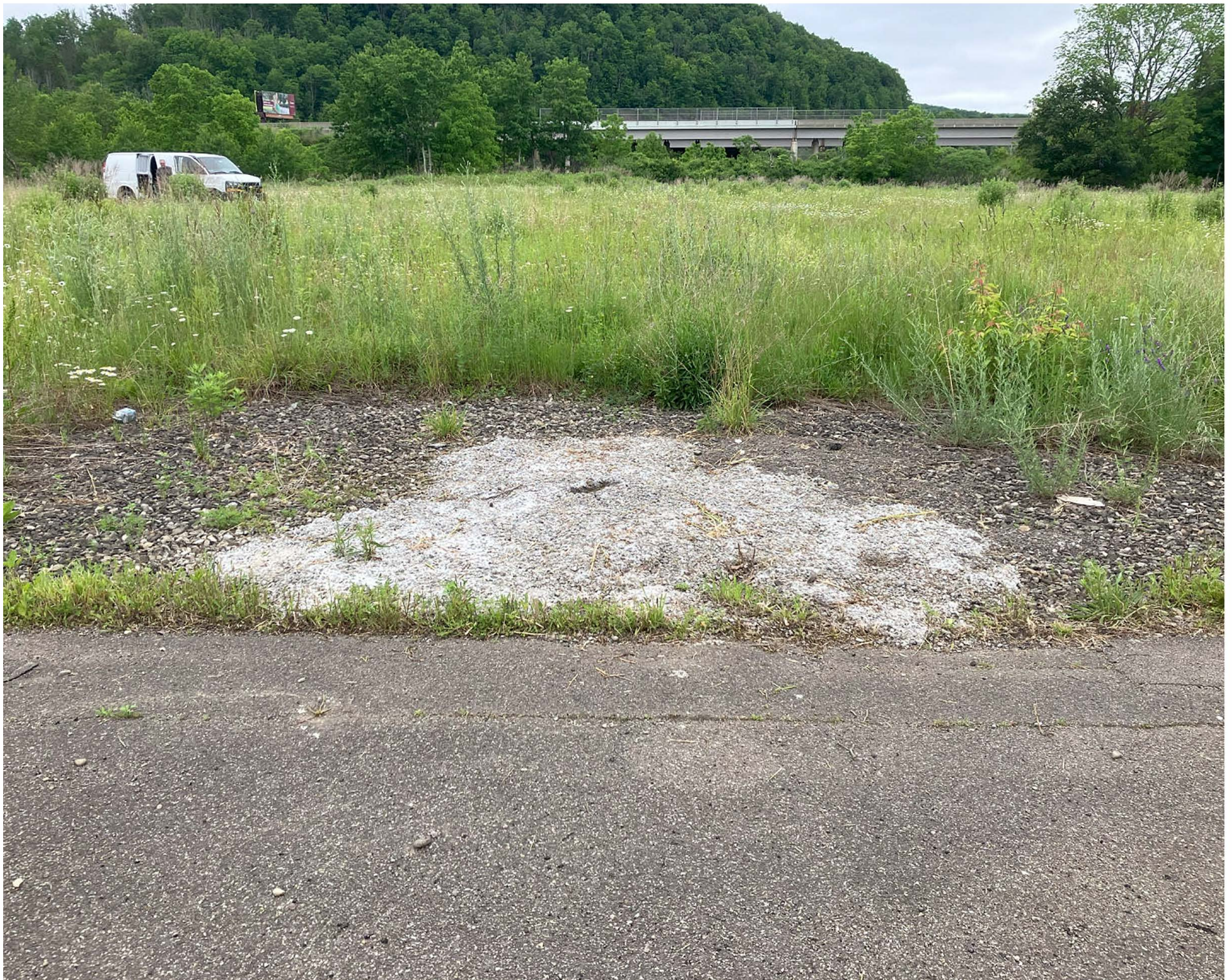
View of a portion of the drainage channel stone cover located along the northern edge of the parking lot, and concrete washout waste, facing northwest.
