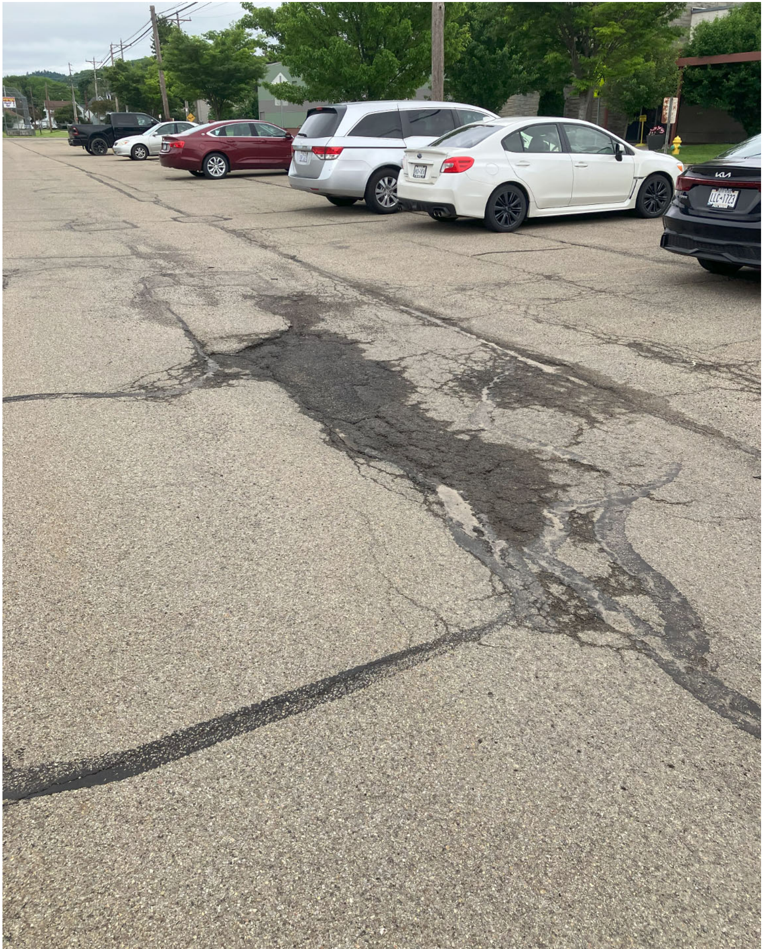
View of an older, deteriorating asphalt pavement patch located in the southern-central portion of the parking lot, facing southeast.
