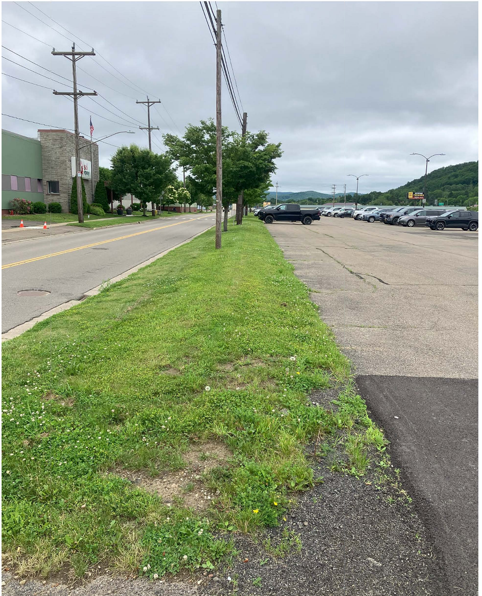
View of asphalt cover (left) and soil cover (right) along the southern edge of the eastern portion of the parking lot, facing west. A poriton of the asphalt repair work (completed October 2024) is visible on the right (foreground).
