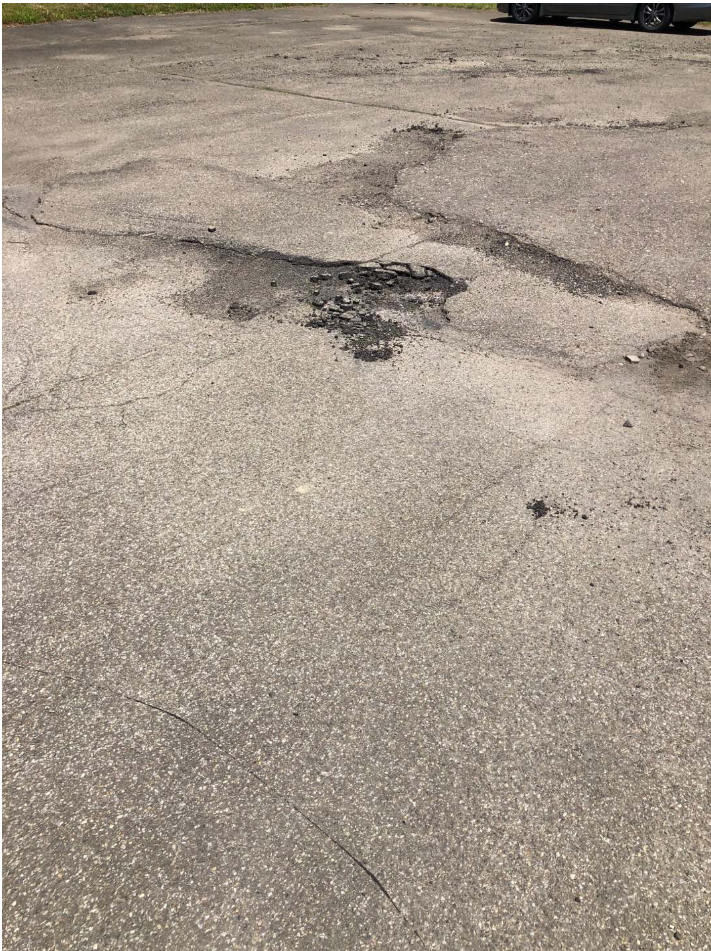
Representative view of broken asphalt pavement in the northeastern portion of the Employee Parking Lot, facing north.
