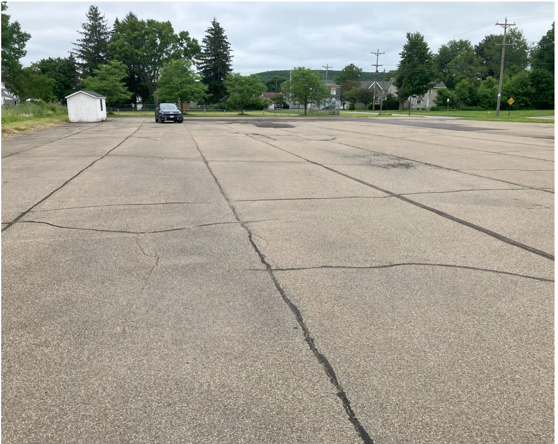
View of the eastern-central portion of the asphalt pavement cover, with older repairs (i.e., sealant along cracks) visible, facing southeast.
