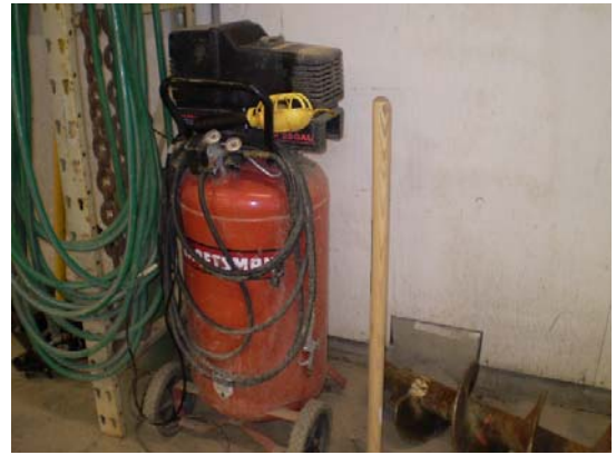
Air compressor within warehouse/storage area of Site building
