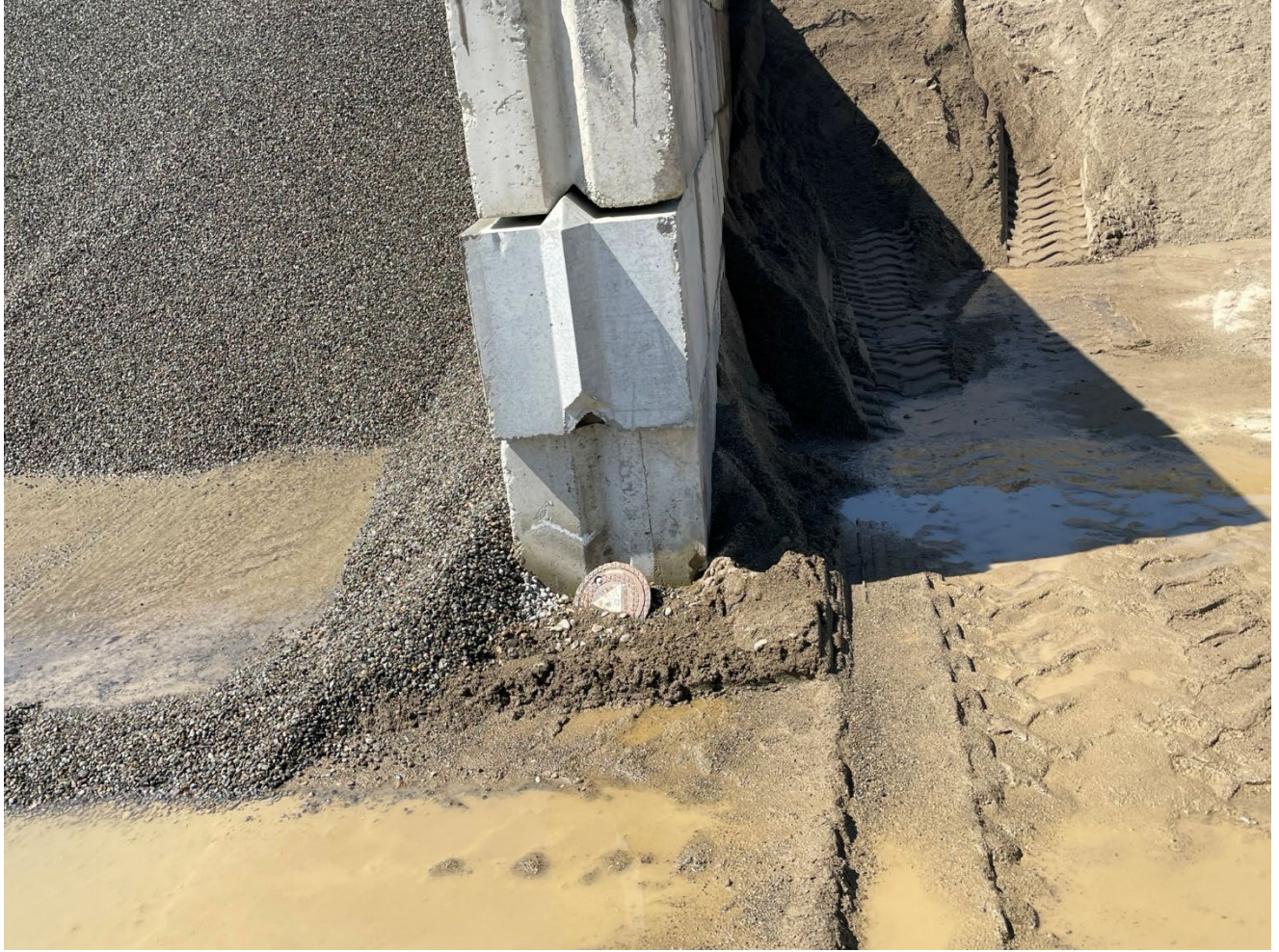
Severed monitoring well cover near materials storage.
