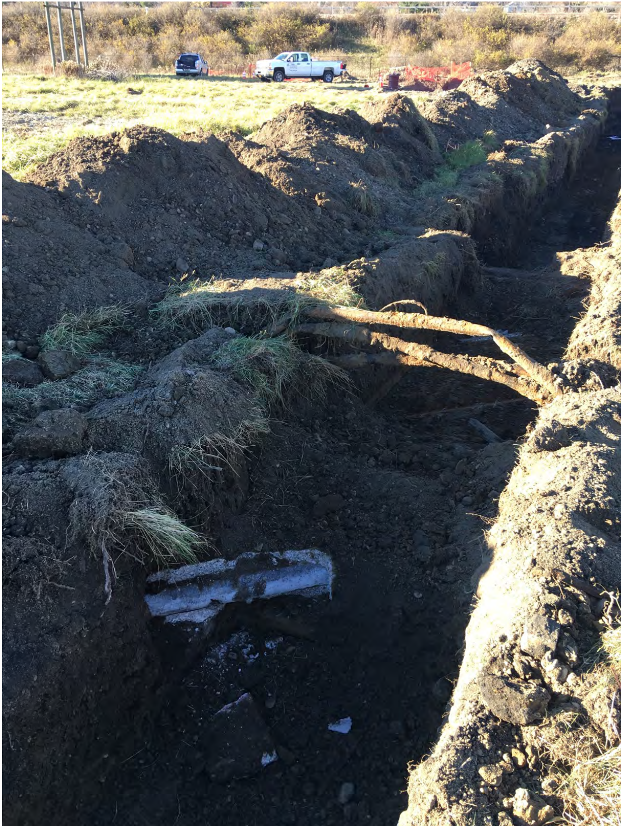
Photo 5: Excavation Zone 3 – 6 pipe cluster at eastern extent of excavation zone (looking North).
