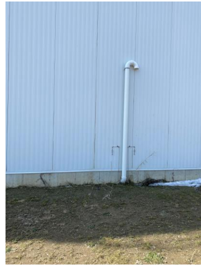
East side Exterior Air Vent
