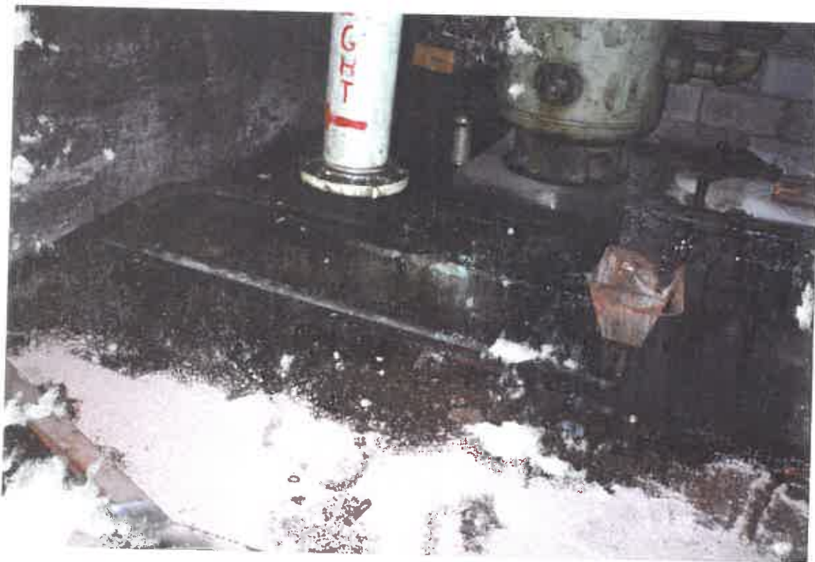
P' .#8: Oil stained floor in building 1A.
