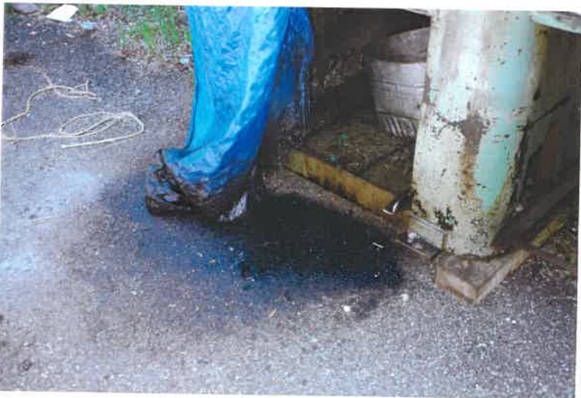
Photo #4: Staining of the parking area, east of the building.
