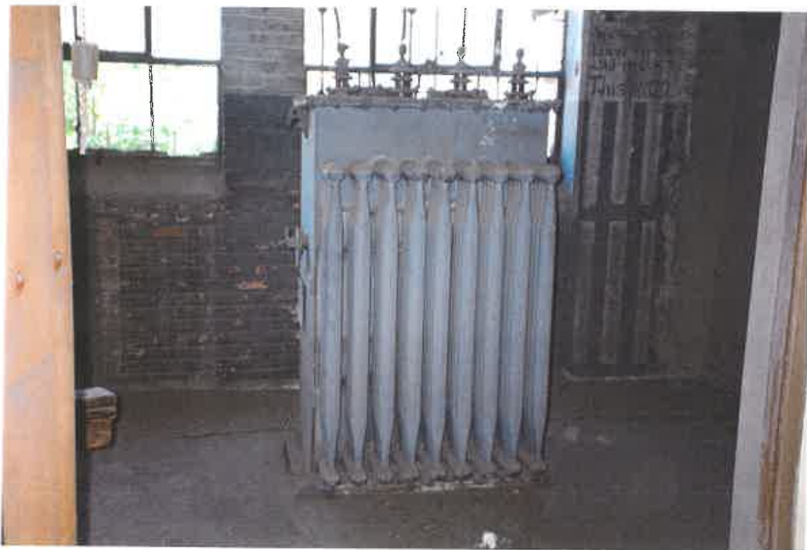
Photo #5: Transformer located on the first floor of building 1A.
