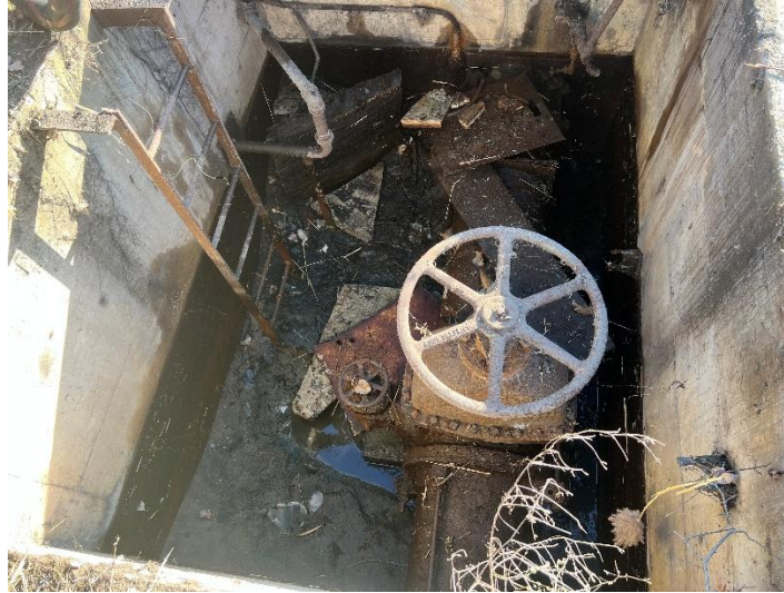
Photograph 1: View from the ground surface look into the valve pit after dewatering was completed. The access ladder is located on the eastern side of the structure.
