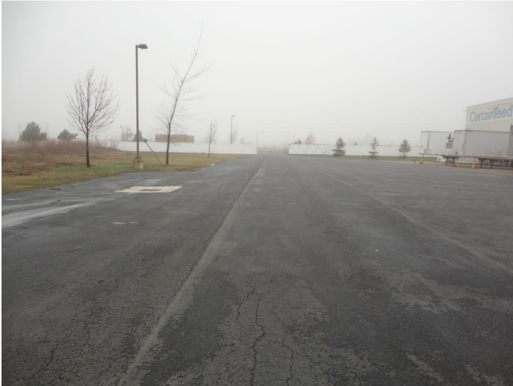
Photograph 3 – at south end of building looking west at new catch basin apron installed 2014
