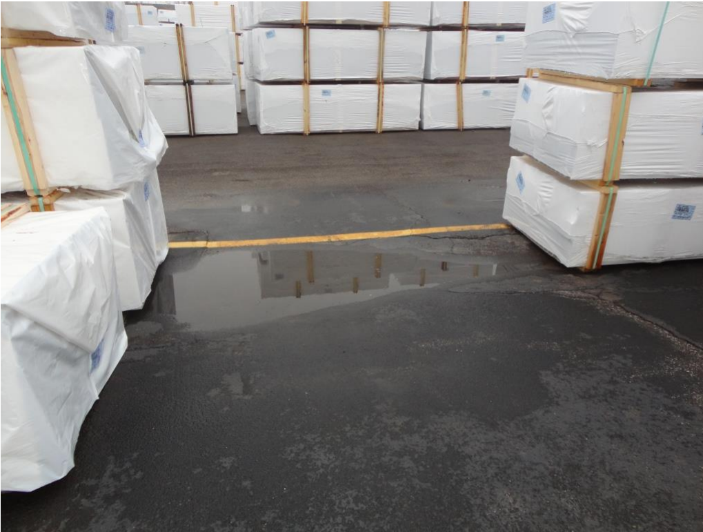
Photograph 16 – Settled/cracked area scheduled for repaving in 2015
