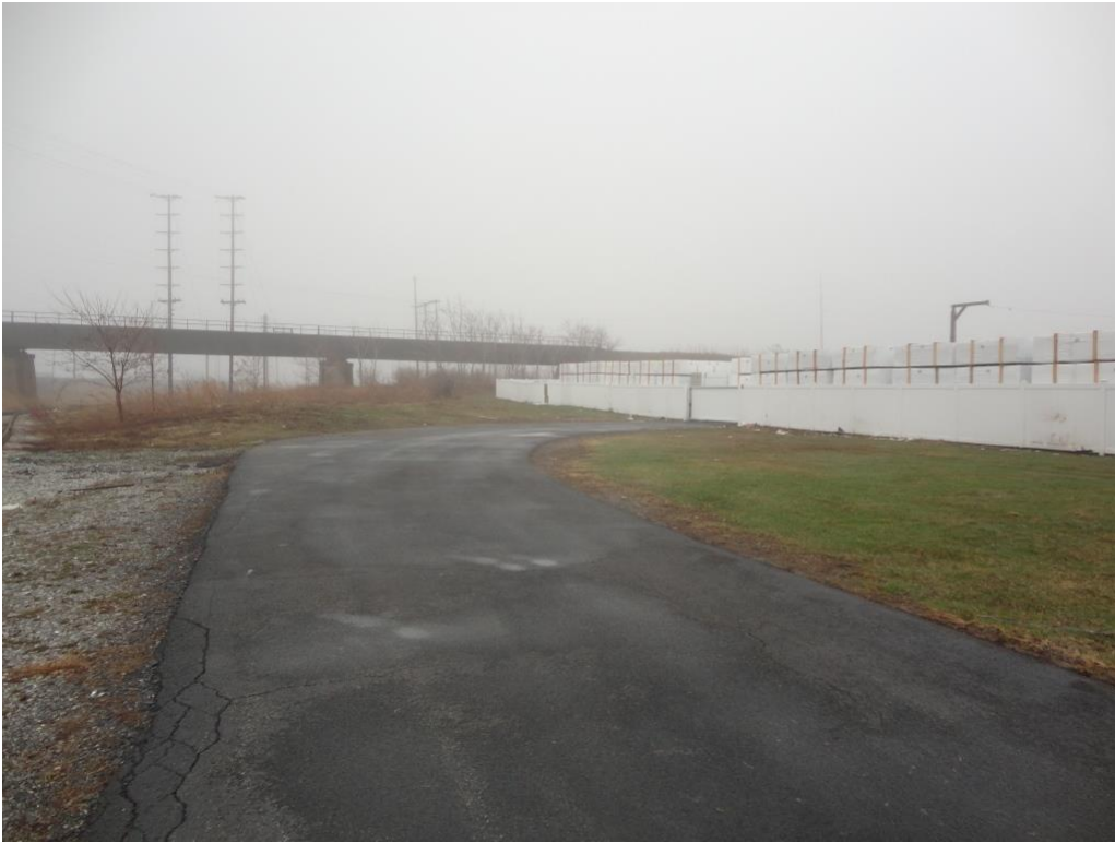
Photograph 13 – Distressed Vegetation on the south side of road and cracked asphalt pavement on the north side of road.
