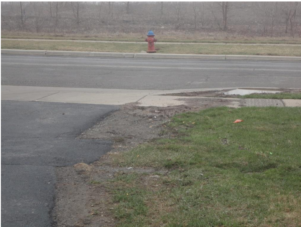
Photograph 6 – Traffic rutting on north side of main entrance apron
