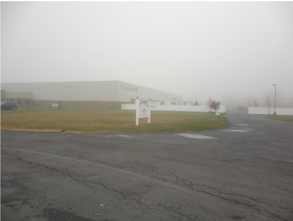
Photograph 14 – Cracked pavement at main entrance
