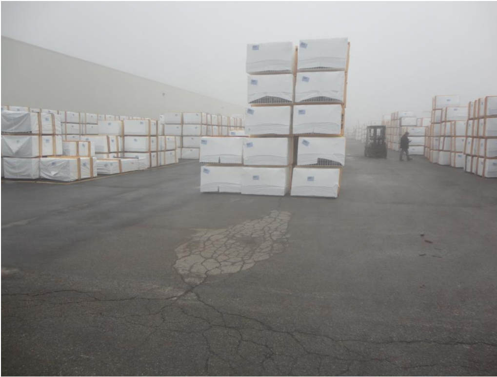
Photograph 15 – Area of cracked pavement in Storage Yard
