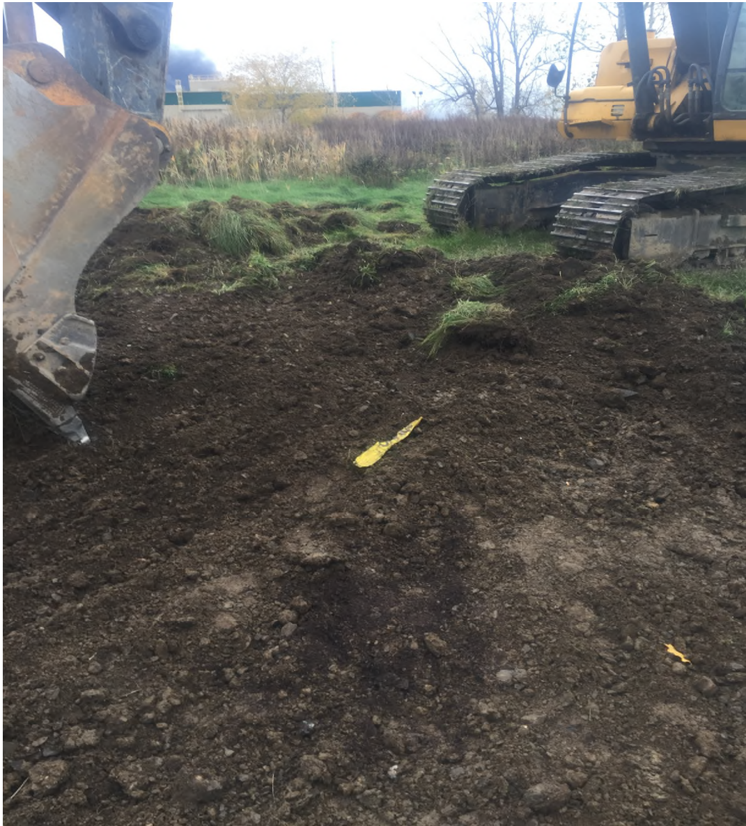
Exposed yellow demarcation tape.
