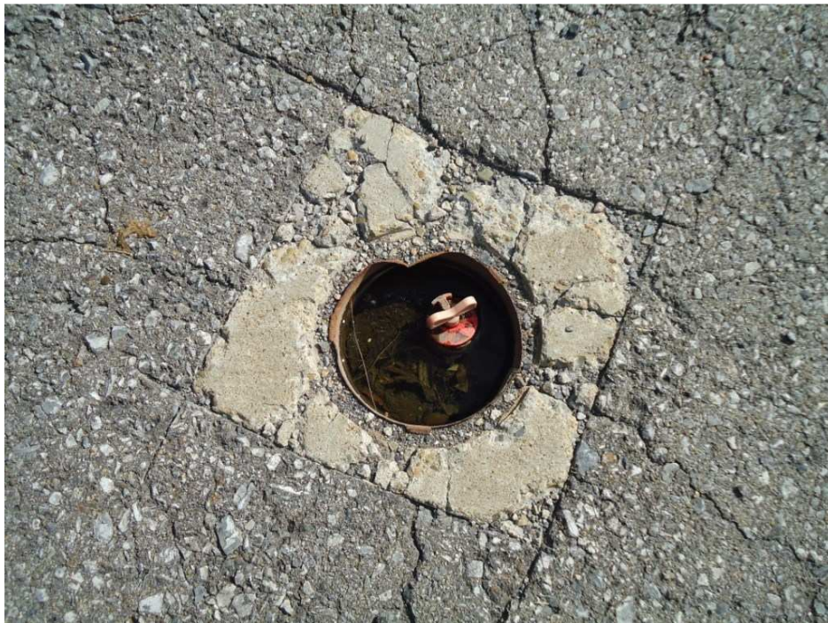
Photo 18 – Damaged casing at MW-106F.
