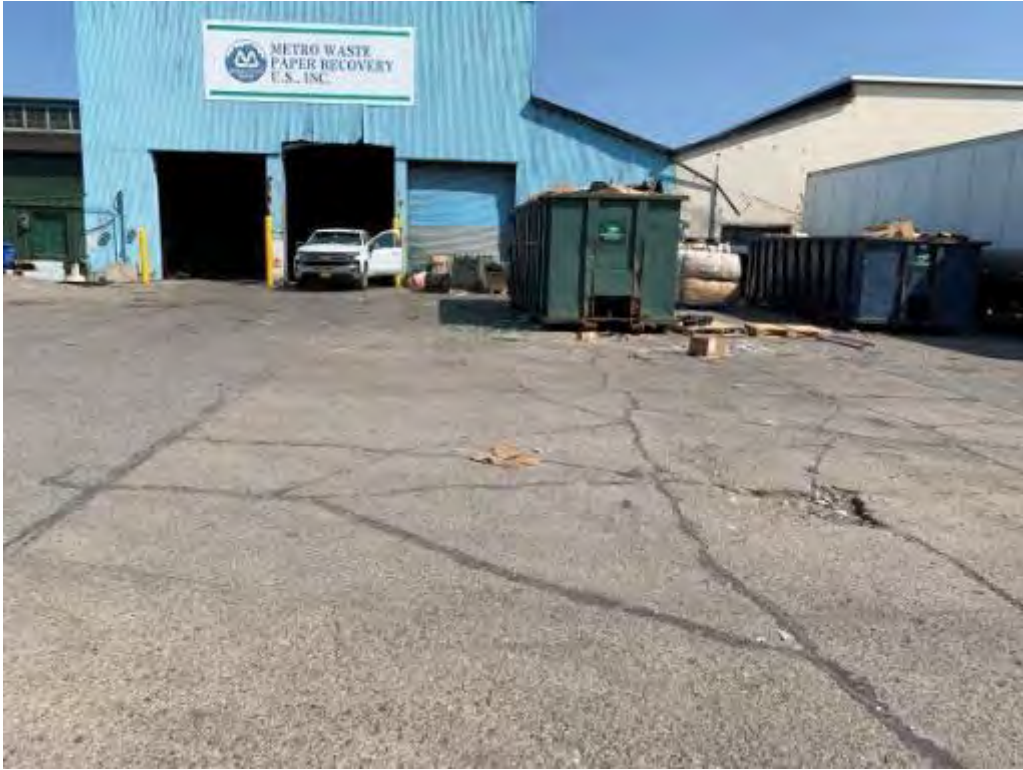
Photo 4 – Building Apron Concrete System (central portion) looking east. Deterioration in right forefront.
