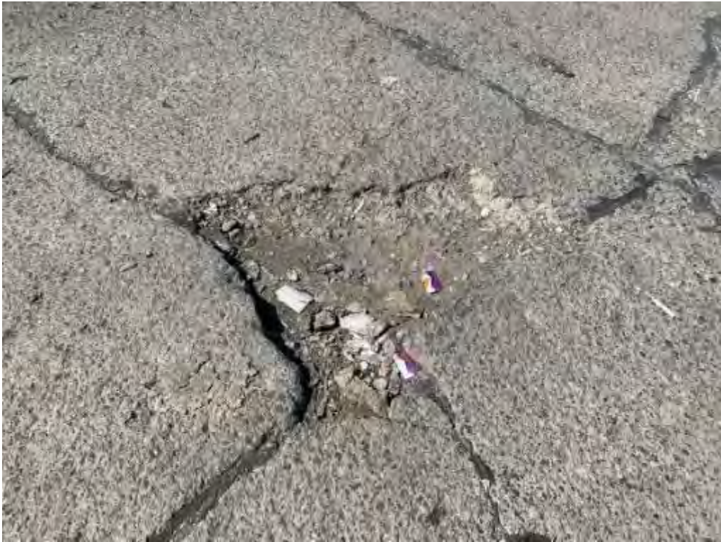
Photo 5 – Closeup of deterioration on central concrete apron.
