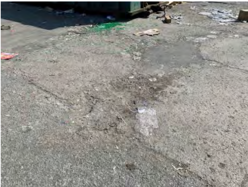
Photo 6 – More deterioration of central concrete apron.
