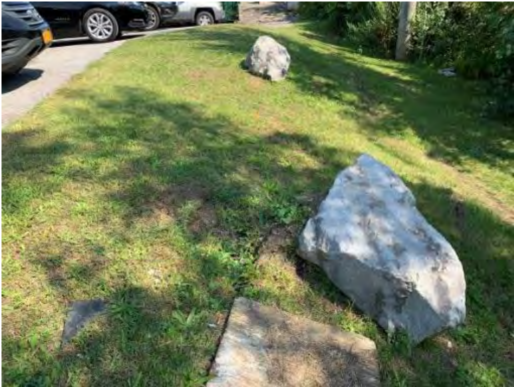
Photo 12 – GCL and Soil Cover System – minor gouging of cover from rock fall.
