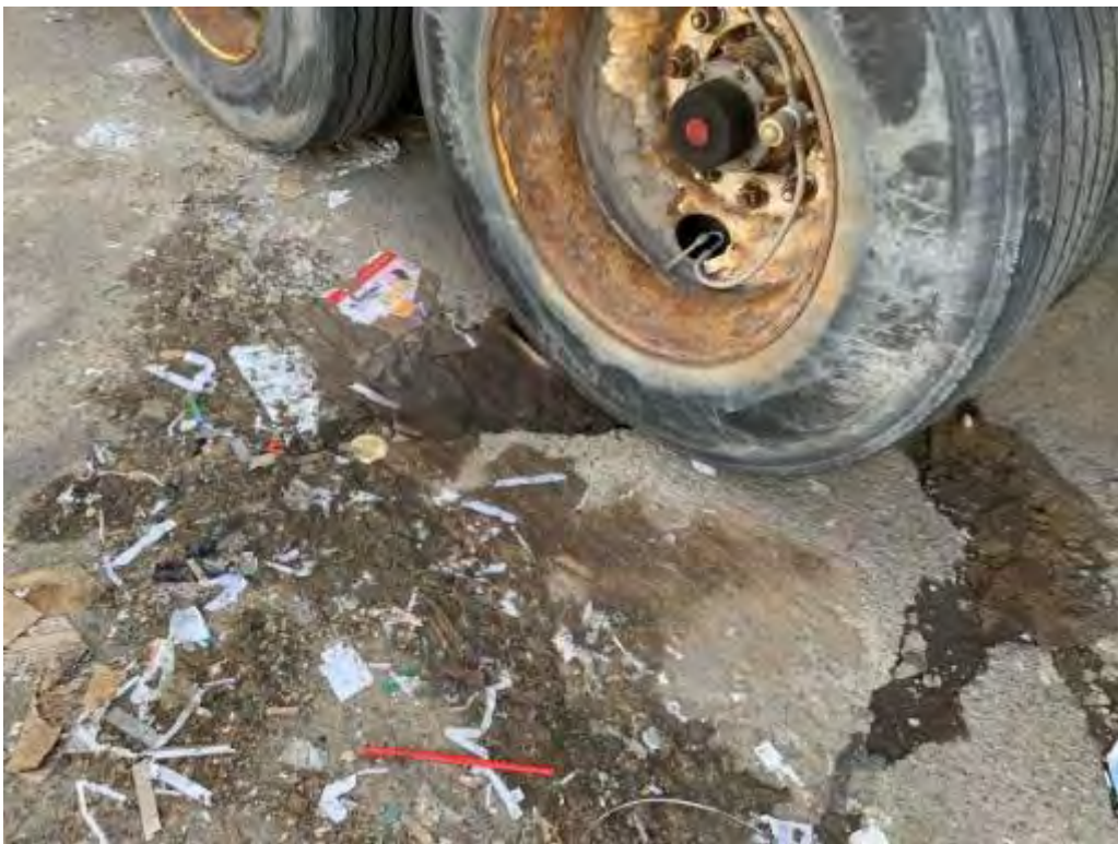
Photo 8 – Deterioration of south concrete apron below truck tires.
