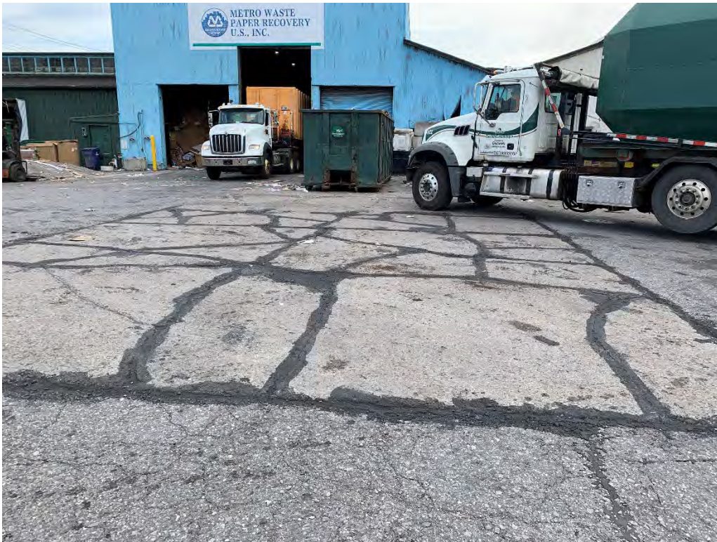
Photo 5 – Building Apron Concrete System (central portion) looking east. Surface cracks are sealed.
