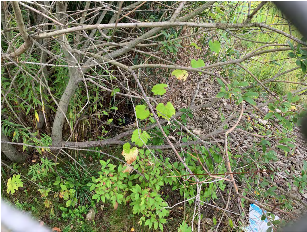
Photo 14 – Looking over outlet pipes of pond.
