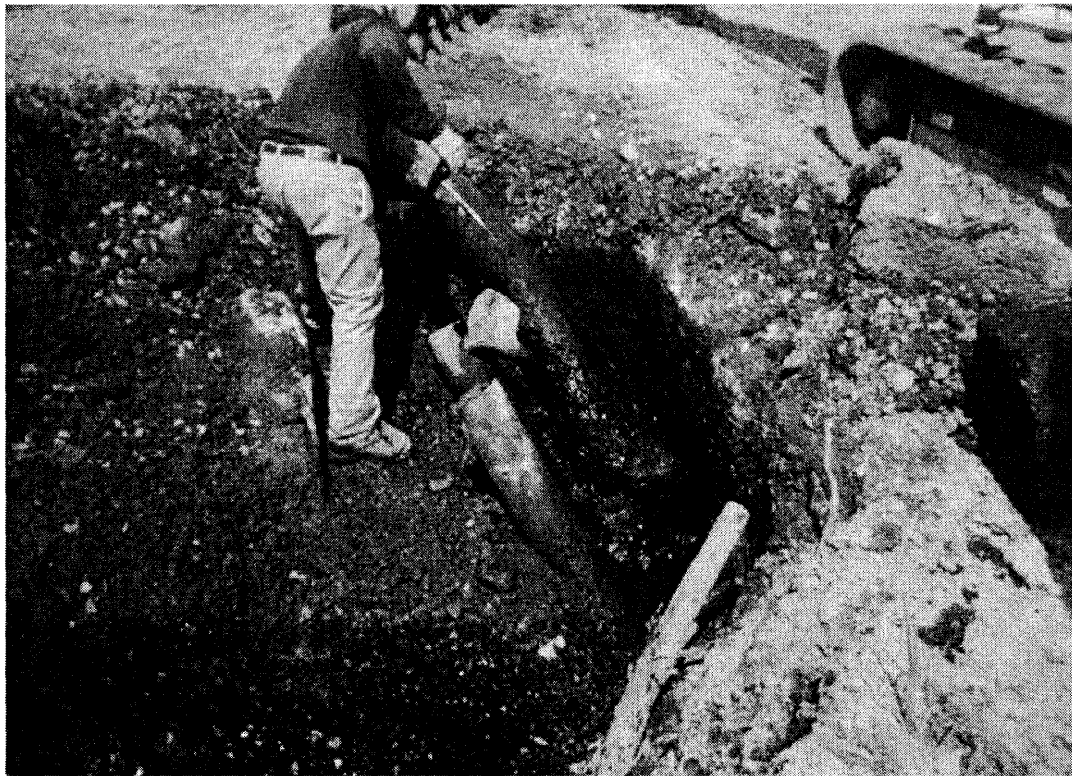
View of TP-10 of pipes entering from the east jutting upwards. The two(2) pipes in foreground are 6" diameter, and one(1) 10" diameter pipe in background. All pipes appear to end at this point. A 3-inch pipe crossing the west side of the trench, aligned north-south cannot be observed.
