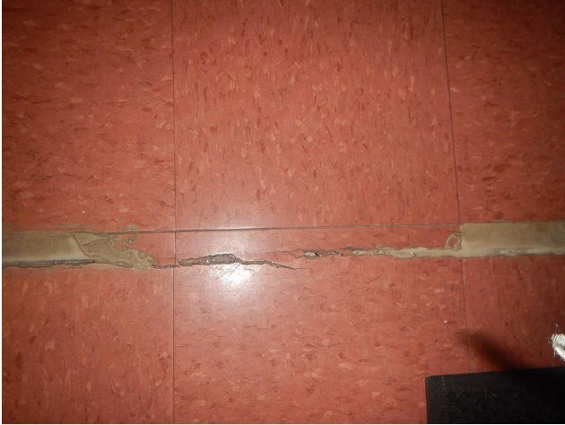
Photo 7: Crack in floor of office hallway
