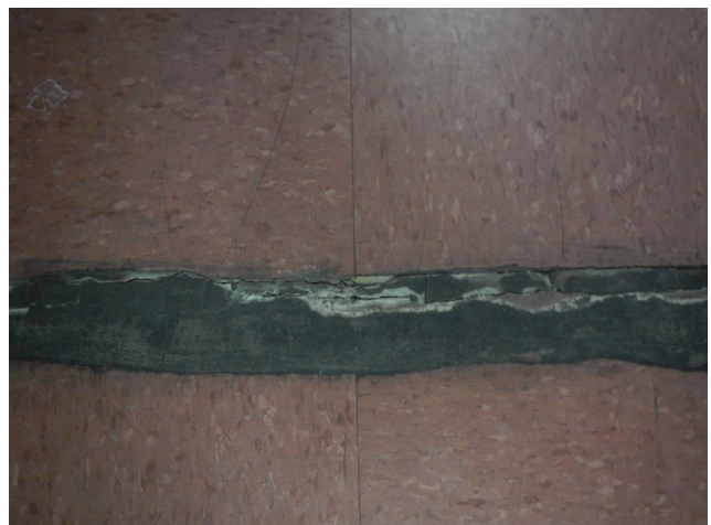
Photo 6: Crack in floor of office hallway
