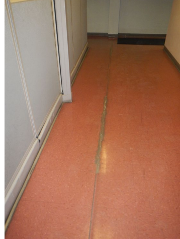
Photo 8: Crack in floor of office hallway
