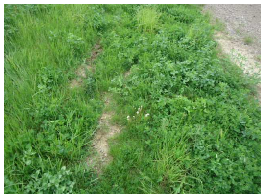
Minor rutting west side of access road between WT-6 and WT-7.
