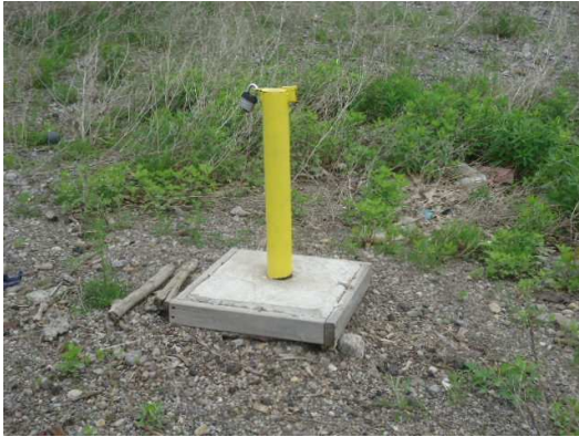
View of soil erosion at monitoring well WT1-05.
