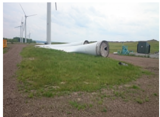
Equipment repair work occurring near WT-6, minor patches of bare vegetation observed.
