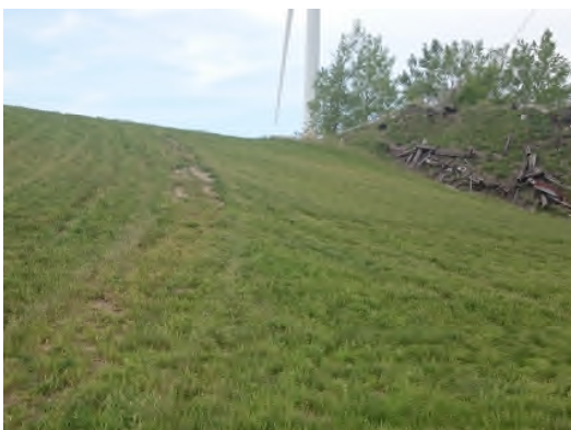
Slight erosion along rut on slope south of WT-8.
