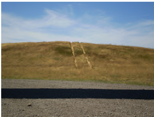
Cover system with evidence of recent vehicular traffic over grassy areas.
