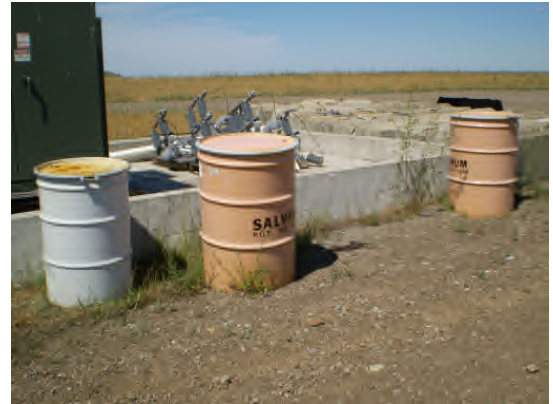
Storage drums of oil impacted grass and gravel staged at area of extra transformer.
