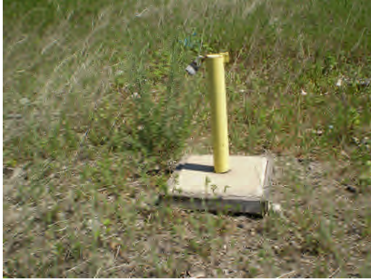
View of monitoring well WT1-05.
