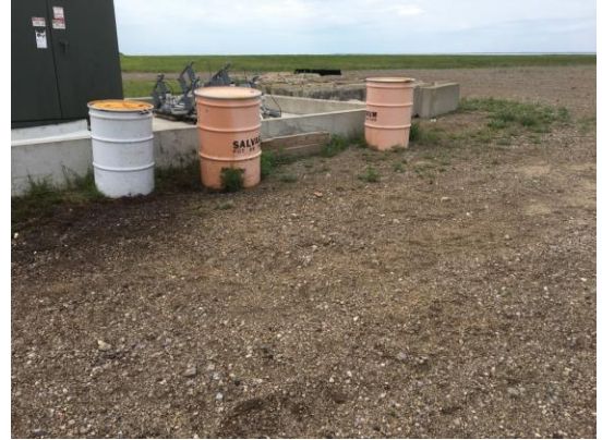
Storage drums of oil impacted grass and gravel staged at area of extra transformer at WT#6.
