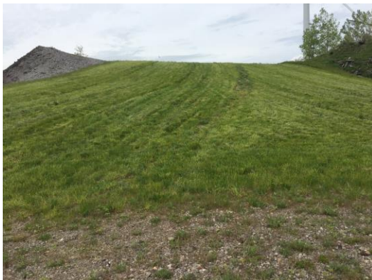
Cover system with evidence of recent vehicular traffic over grassy areas, looking northerly towards slope up to WT#8.
