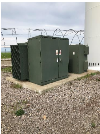
View of WT 3 electrical transformers.
