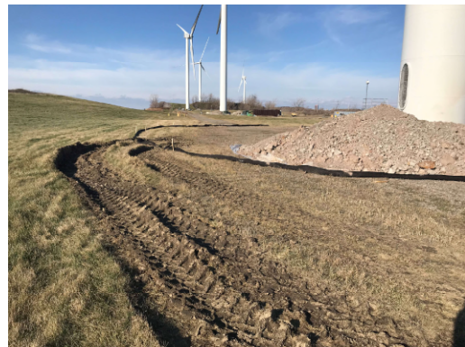
Photo 6: View of soil cover rutting from construction equipment.
