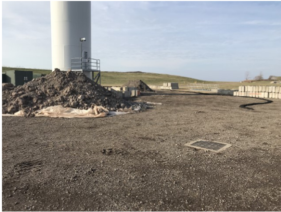
Photo 1: Turbine 5 work location with missing erosion control wattle. Note nearby storm drain.
