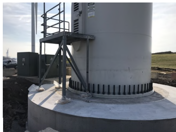
Photo 6: View of Turbine 5 with new concrete foundation. Note installation of elevated platform.
