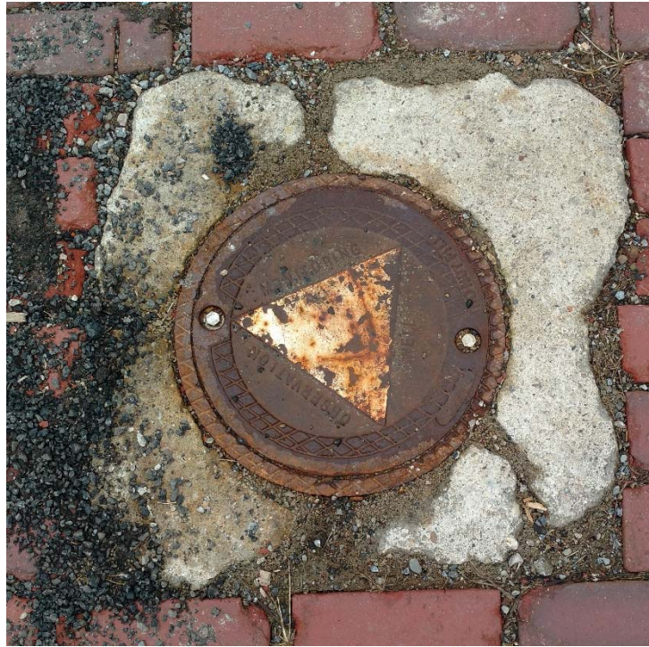
Injection well IW-24, cracks in concrete collar.
