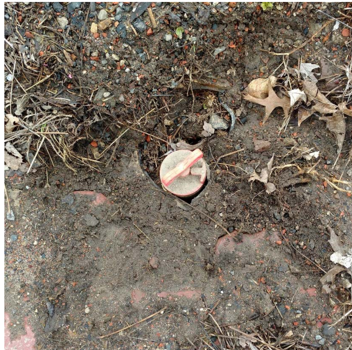
Monitoring well MW-11, damaged curb box.
