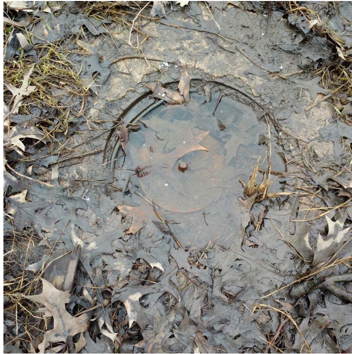
Monitoring well MW-22A, damaged curb box.
