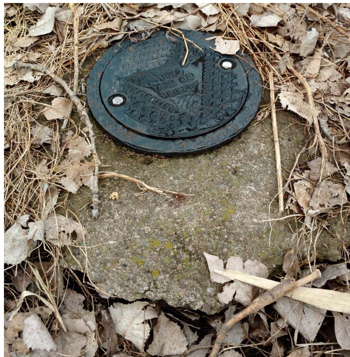
Monitoring well MW-9A, undercutting of concrete collar.
