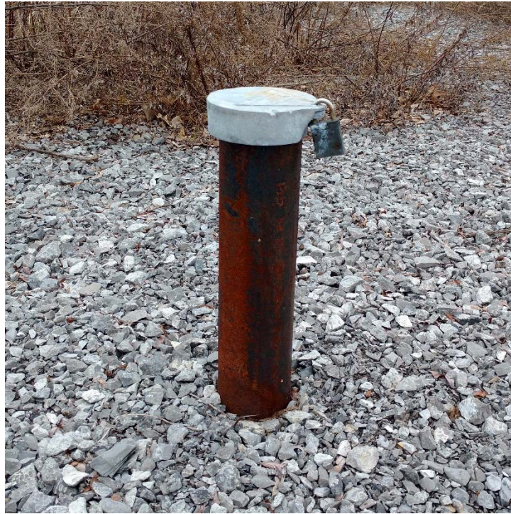
Injection well IW-4, loose cap.
