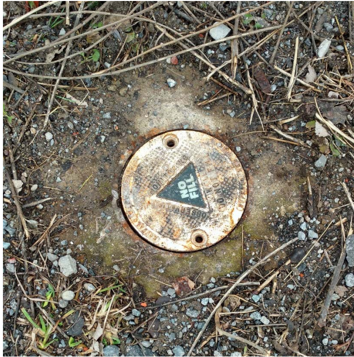
Monitoring well MW-7, missing 2 lid bolts.
