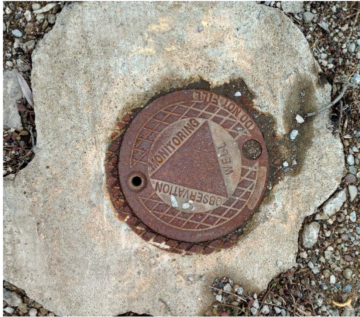
Monitoring well MW-20A, missing 1 lid bolt.
