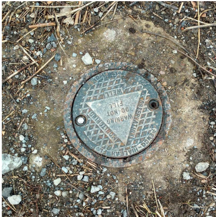
Monitoring well MW-7A, missing 1 lid bolt and j-plug.
