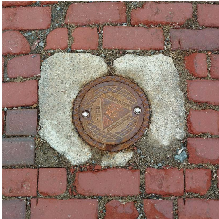
Injection well IW-26, cracks in concrete collar.
