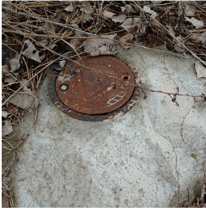
Monitoring well MW-9, missing 1 lid bolt.
