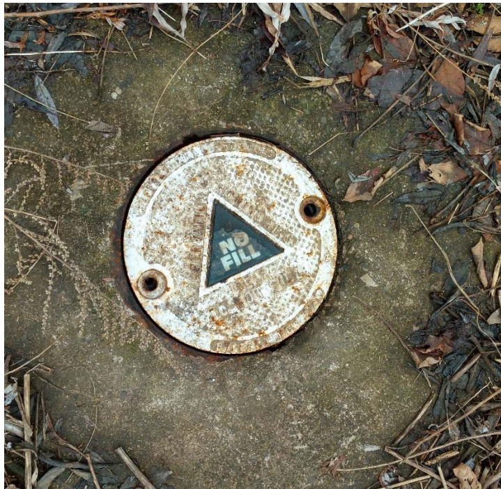
Monitoring well MW-6, missing 2 lid bolts.
