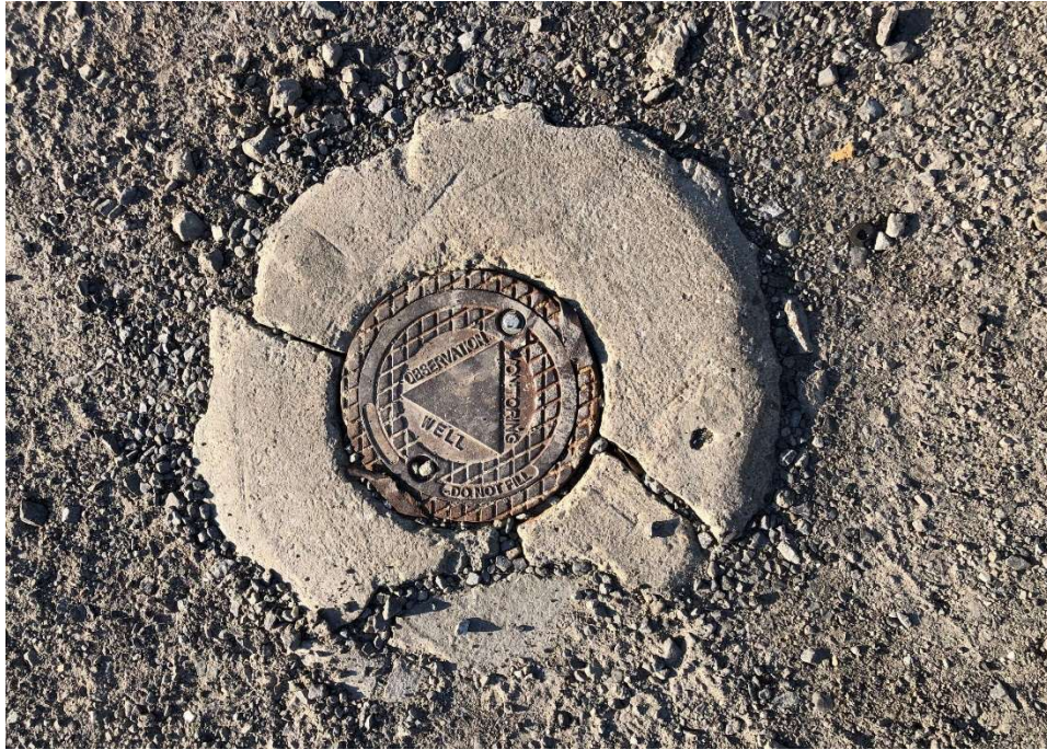
Typical cracked concrete road boxes (see inspection form for list of wells).
