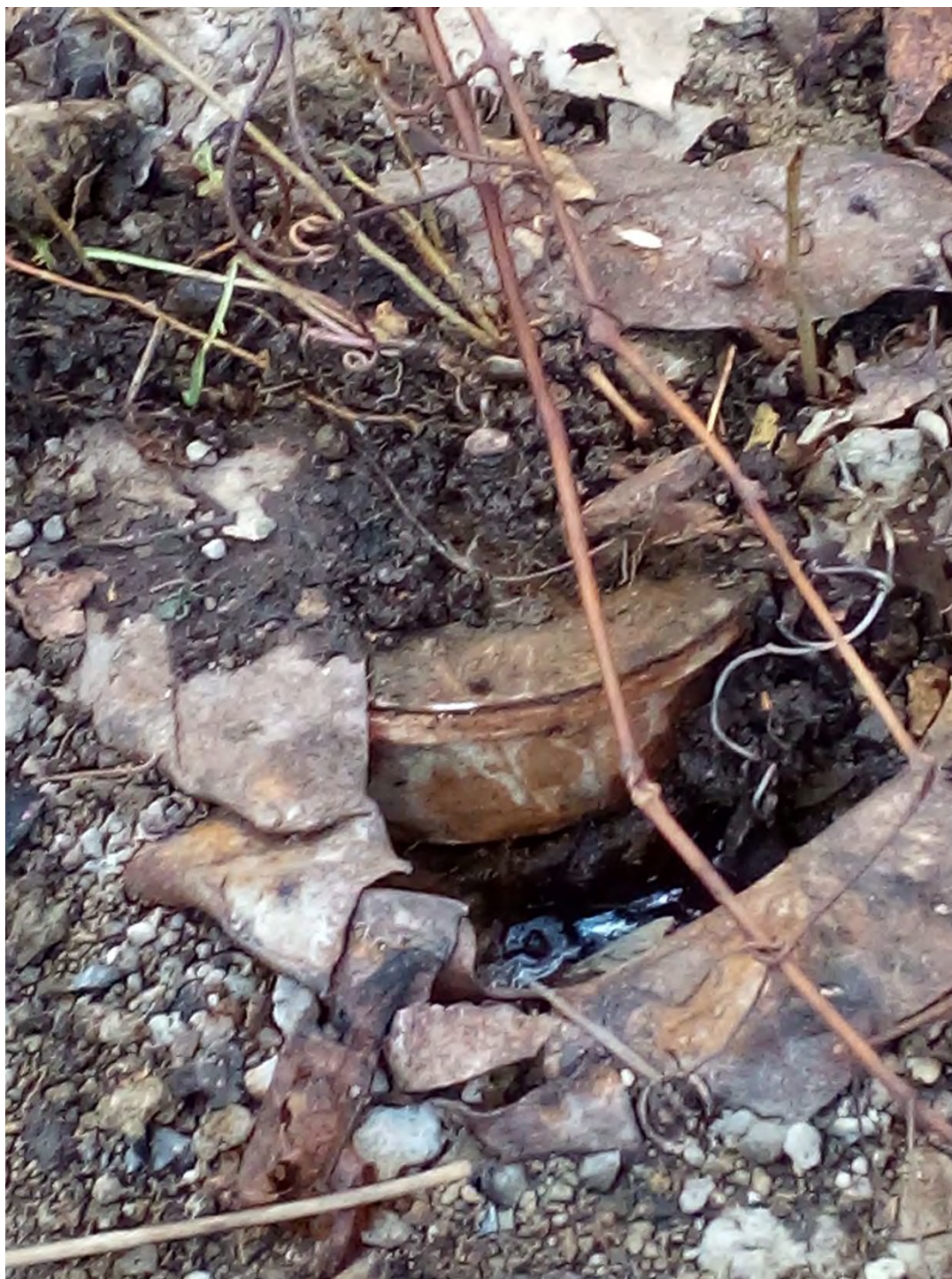
Damaged curb box at monitoring well MW-7A.
