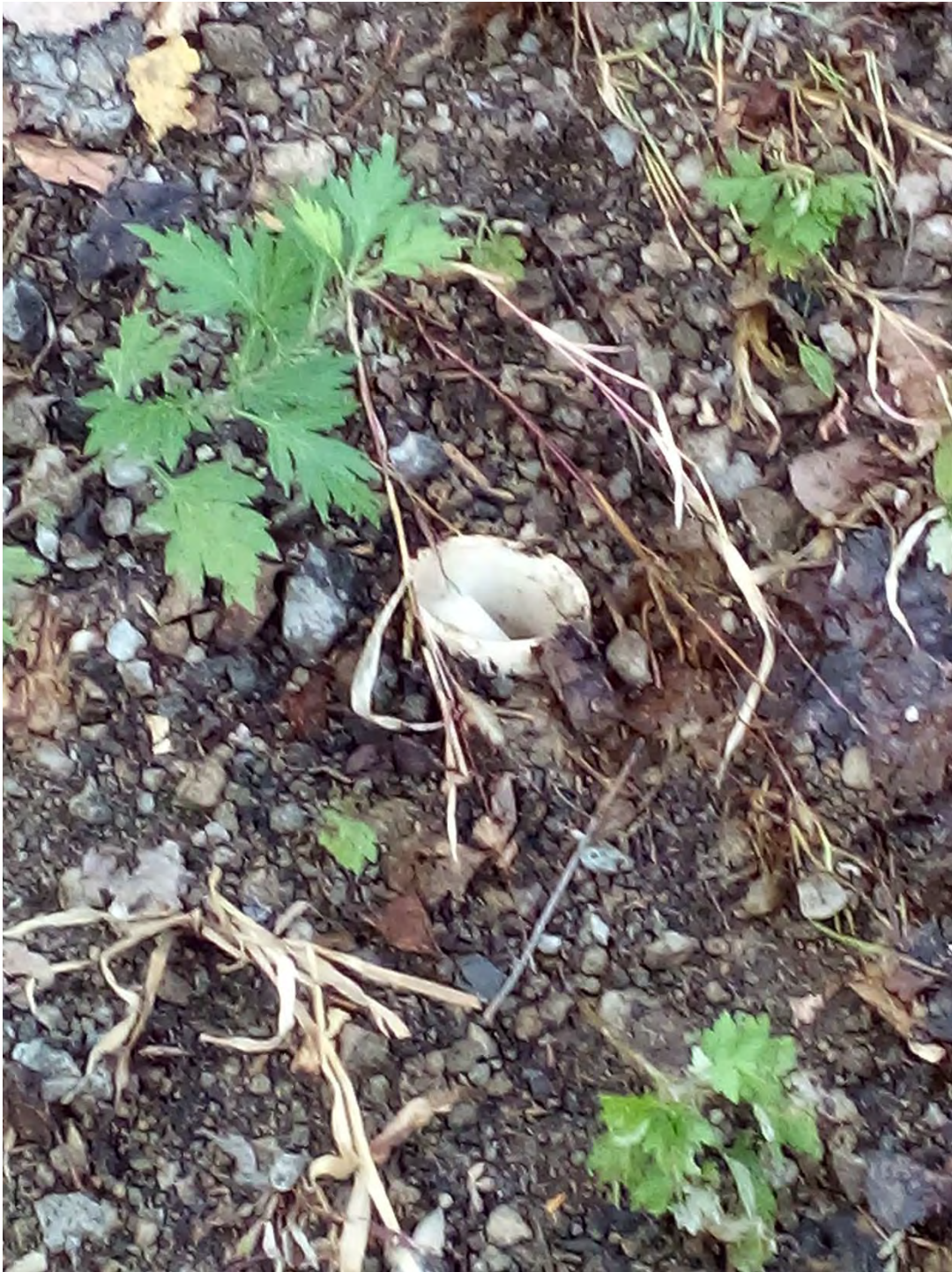
Missing curb box and damaged PVC casing at monitoring well MW-7.
