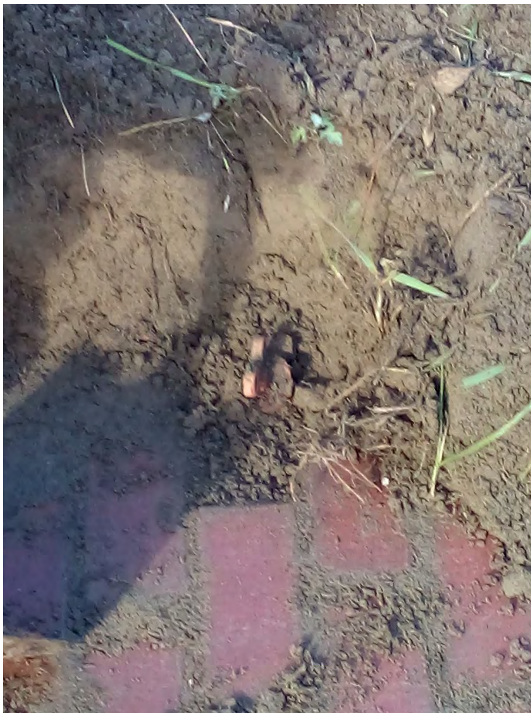
Missing curb box at monitoring well MW-11.
