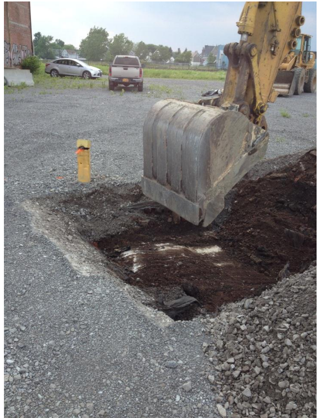
Concrete Foundation Refusal Near RFI-31
