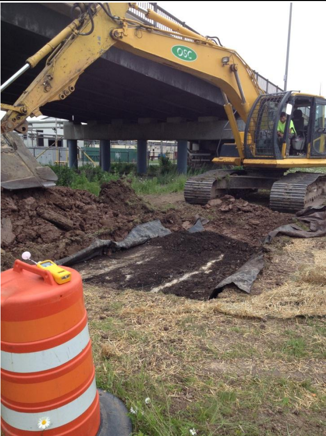
Concrete Foundation Refusal Near RFI-20
