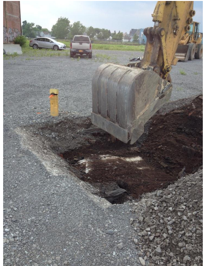
Concrete Foundation Refusal Near RFI-31
