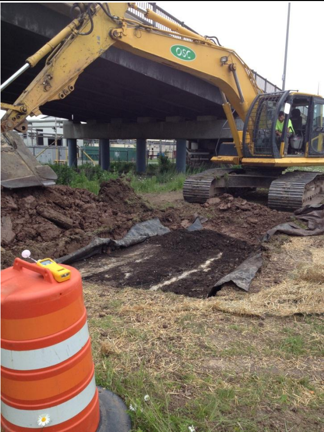
Concrete Foundation Refusal Near RFI-20
