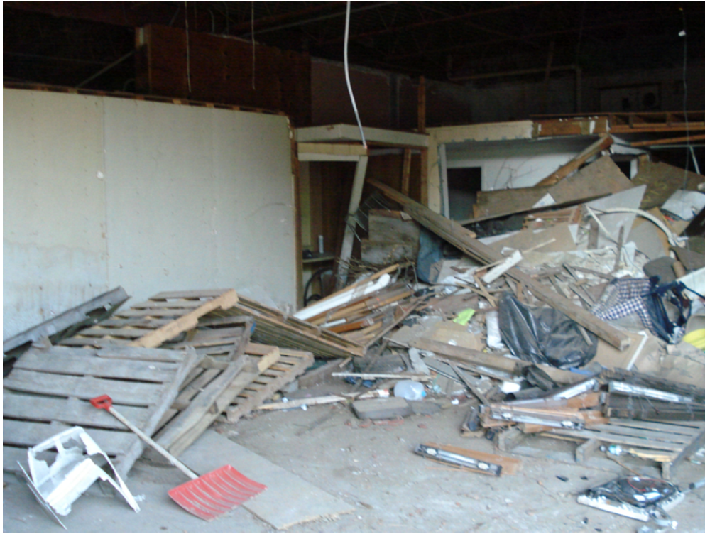
Typical pile of debris in Building 3
