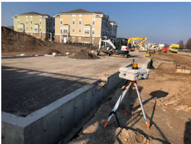
Dust monitor station looking west
