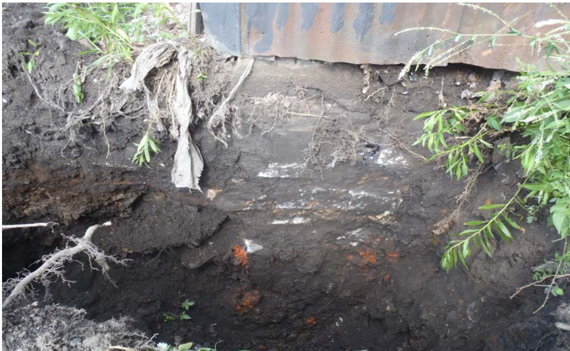
Photograph 4 –Test Pit TP-3 –Stone Block and Possible Brick Foundation Wall – Falling Apart
