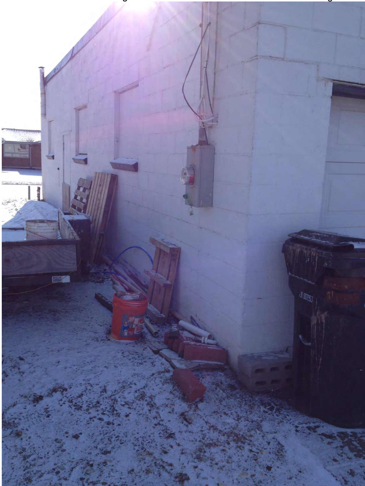
Photo 4: View of debris along the northern exterior wall of the Eastern Building
