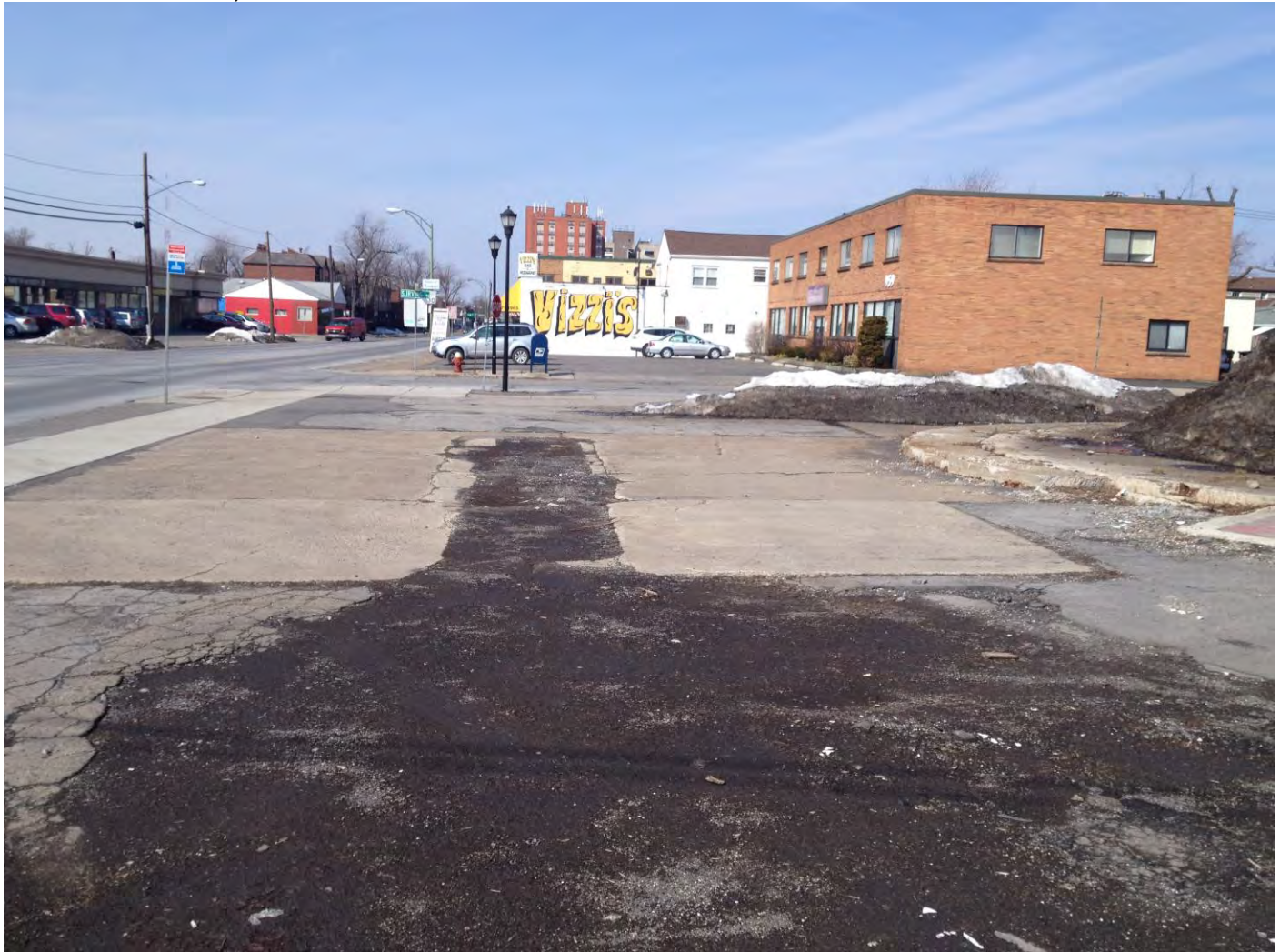
Photo 22: View of a former pump island south of the former Western Building (looking west)
