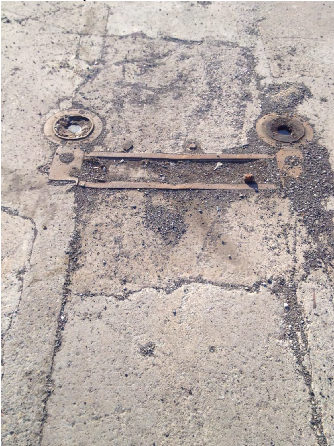
Photo 21: View of a historic in-ground hydraulic lift in the footprint of the former Western Building
