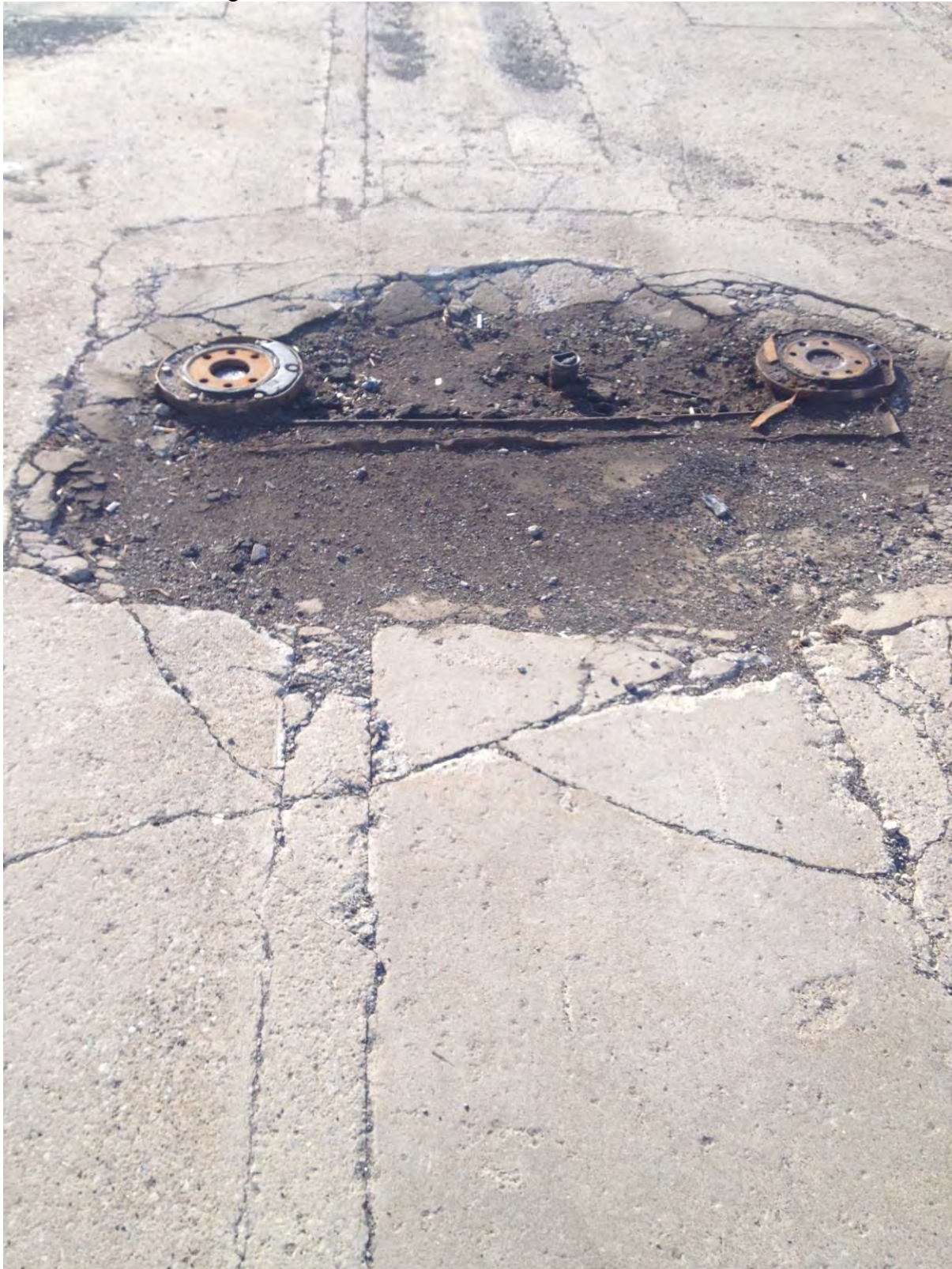
Photo 19: View of a historic in-ground hydraulic lift in the footprint of the former Western Building
