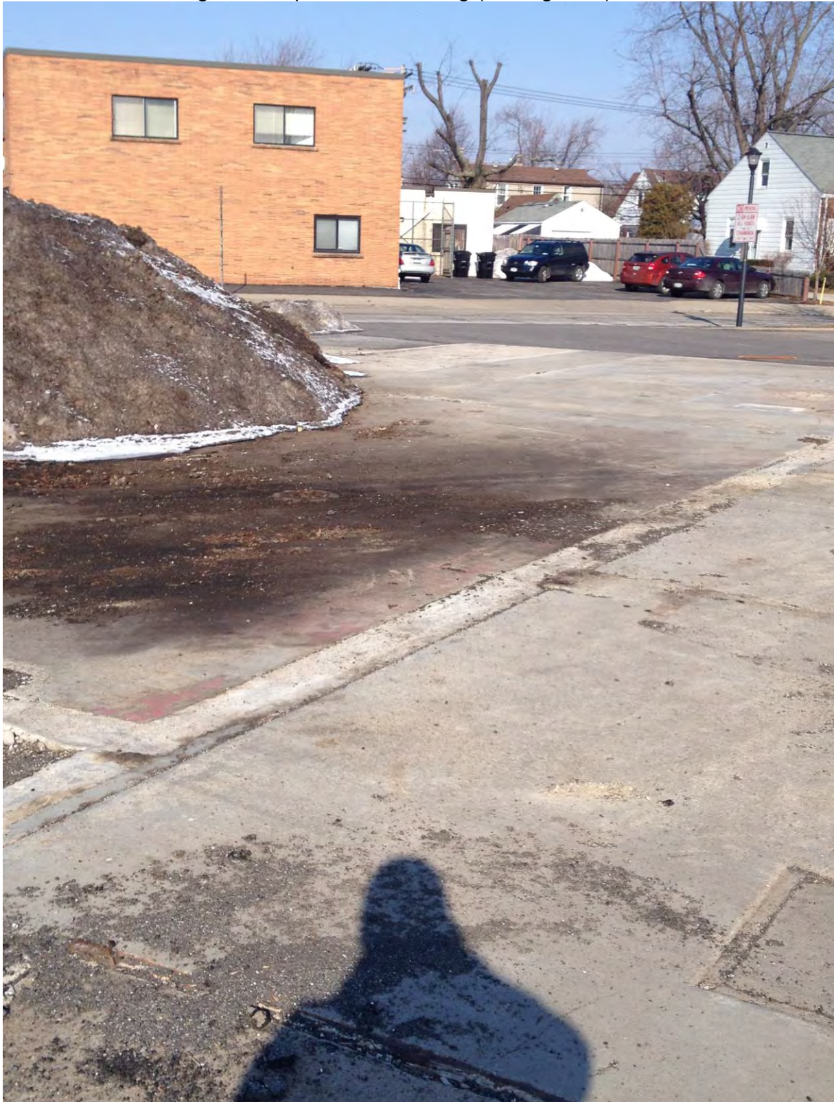
Photo 18: View of 1 historic in-ground hydraulic lift in the footprint of the former Western Building with suspected oil staining (looking west)
