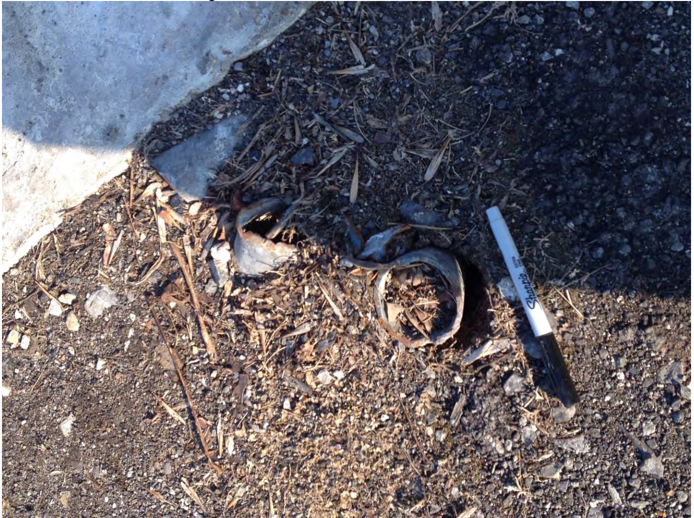
Photo 16: View of 2-3 suspected cut vent pipes on the southeastern edge of the former Western Building
