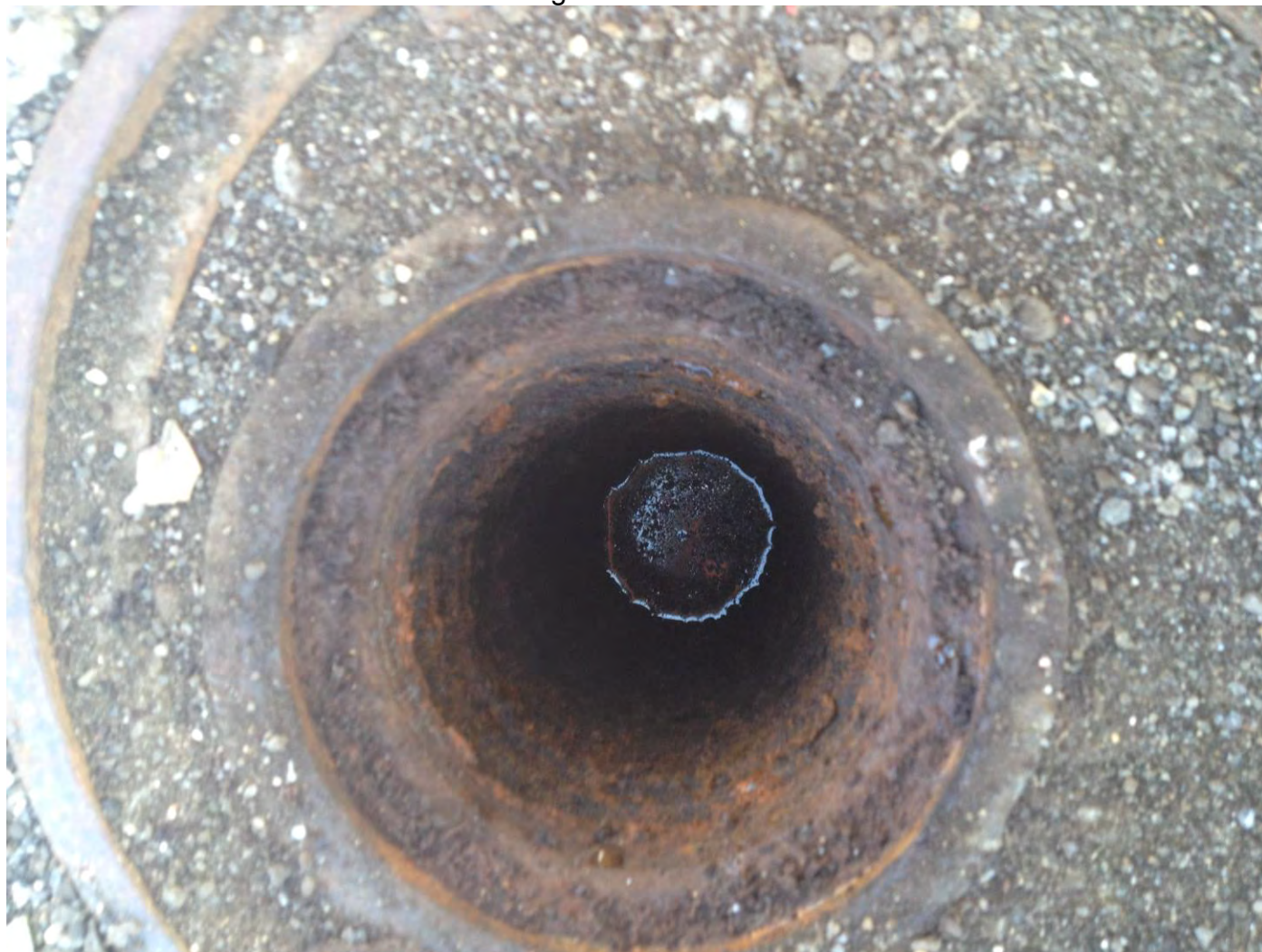
Photo 12: View of water in the UST associated with the fill port on the northwestern edge of the former Western Building
