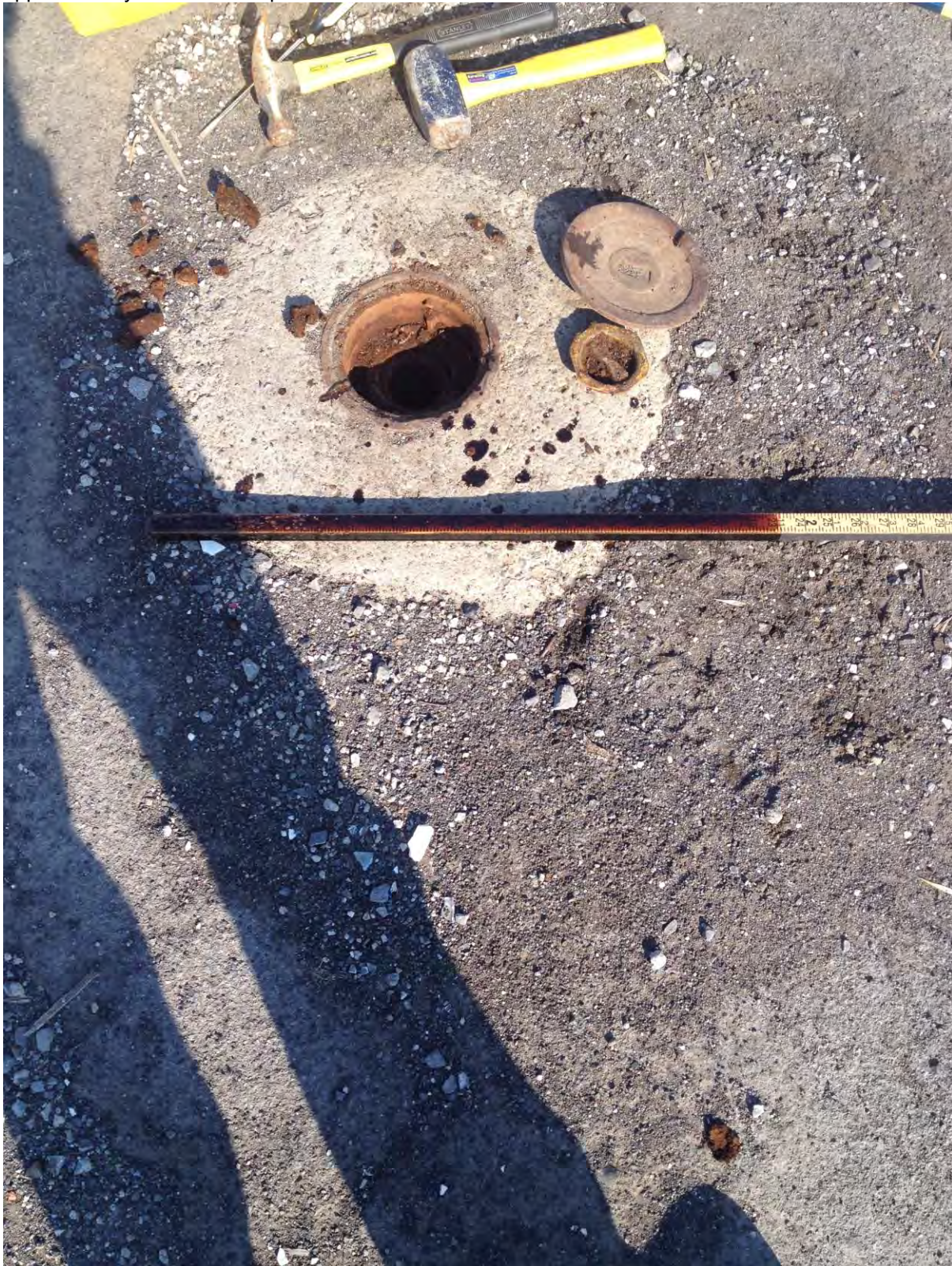
Photo 15: View of the opened fill port on the southeastern edge of the former Western Building and approximately two feet of oil product from the associated UST
