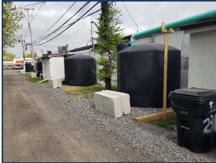
Photo 5 – View of the water cistern system behind the building.
