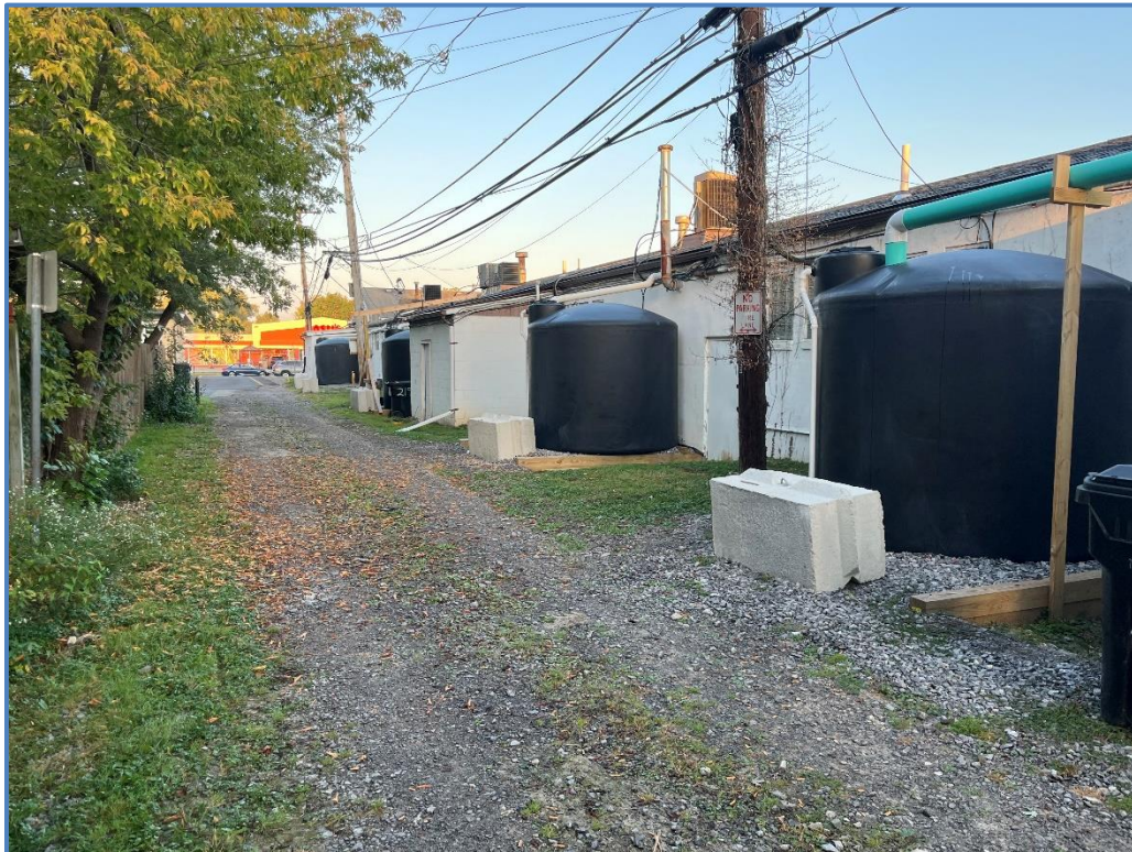
Figure 6-13. Photo showing the storm water management system behind Highland Plaza. View looking west. Precipitation from the roof of the plaza is diverted through piping to four large poly tanks. Water is then conveyed from the tanks to the storm sewer system along Colvin Boulevard. Photo taken by Glenn M. May October 4, 2023.
