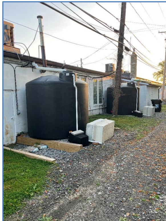
Figure 6-14. Photo showing tanks 1 and 2 of the storm water management system. View looking east. Photo taken by Glenn M. May October 4, 2023.
