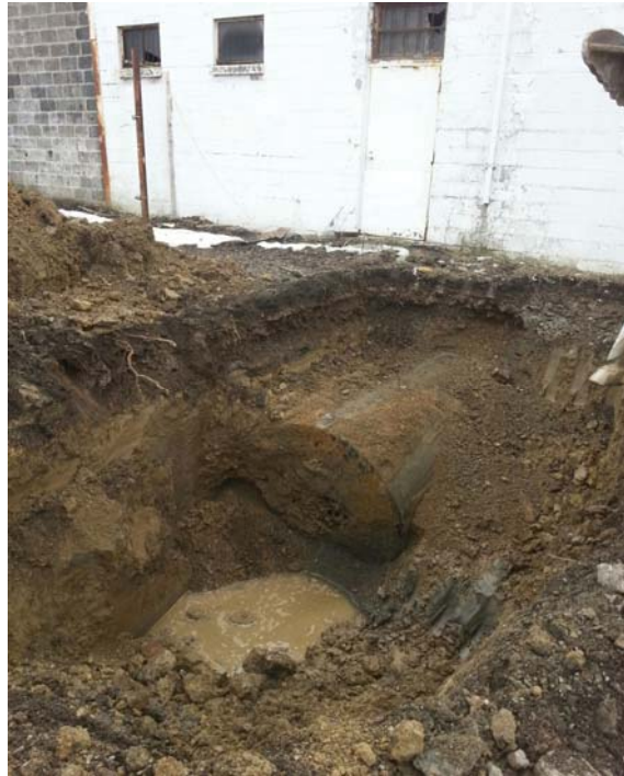
Photo #1 - Abandoned UST in-place
