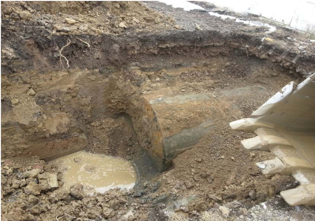
Photo #2 - Abandoned UST in-place
