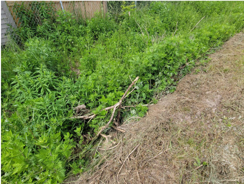
Photo #10: Debris in drainage ditch bordering houses along southern boundary.
