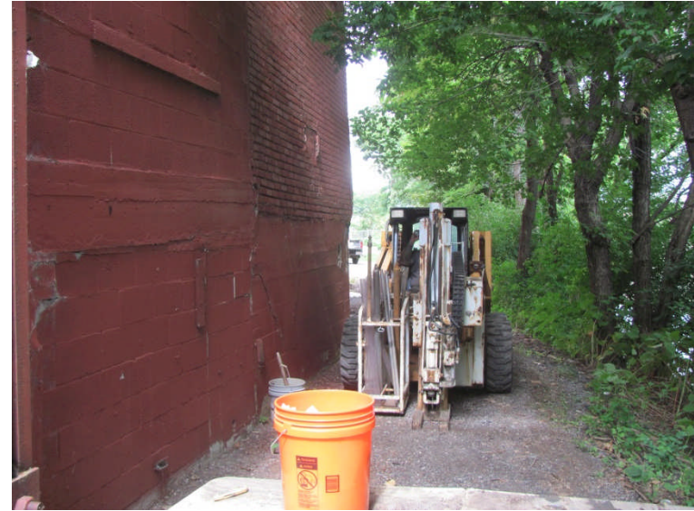
42. Location of borehole BH5-1n facing north; 15 feet north of phase 2 borehole BH-5
