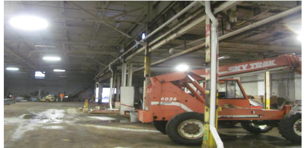
8. View of SSDS piping
