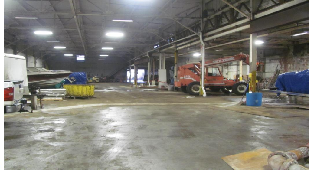
6. High-Bay area SSDS vertical piping
