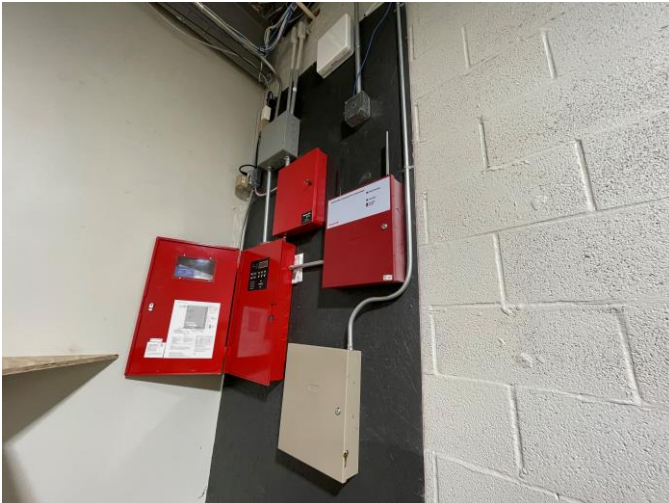
View of vapor system control and fuse box.
