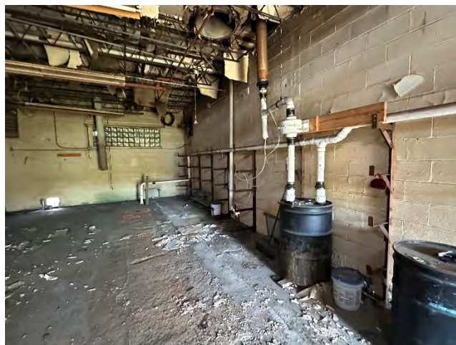
Photo 4: Former SVE System installed within 1746 Dale Road Metal Prep Building; looking northwest. Carbon vessel (center right) and one of two extraction wells (against back wall).
