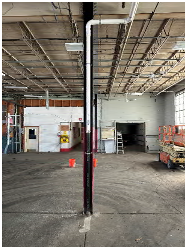
Photo 6: Existing SSDS piping within 24 Anderson Road Building; looking east.
