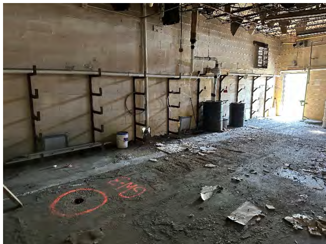
Photo 5: Former SVE System within 1746 Dale Road Metal Prep Building; looking northeast. Monitoring well GW-3 (at left) and second extraction well (far right).
