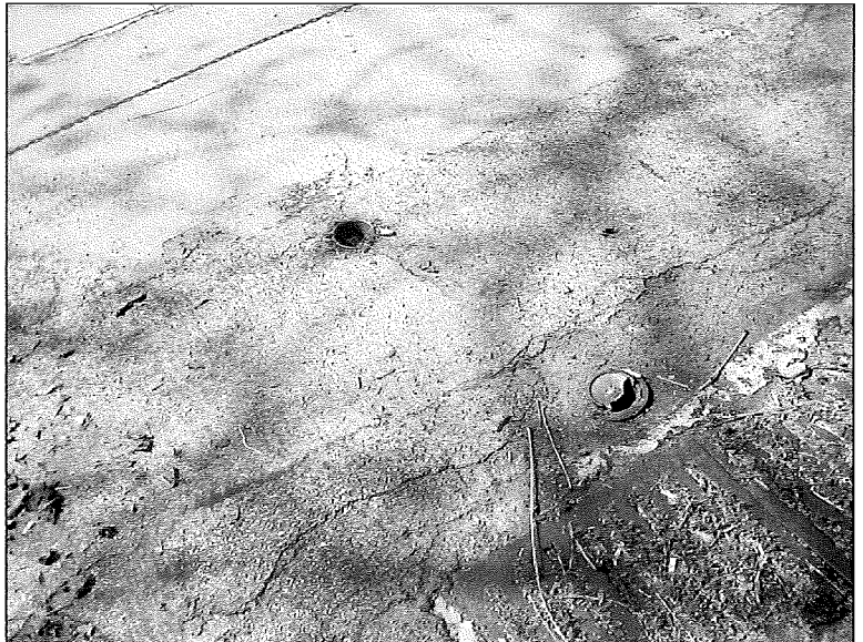
Sewer vent and cleanout
