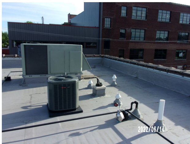
2. View of RT-1(061422) located on the roof of the ciderly near the air intake for the HVAC system.
