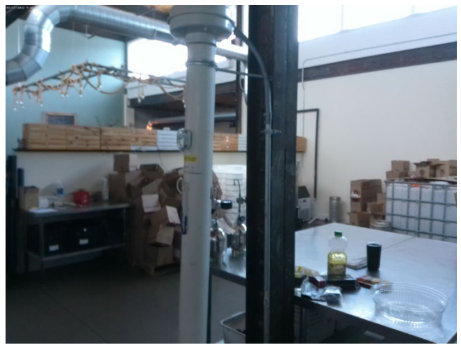
10. 12/19/22 – View of SSDS #4 Piping
