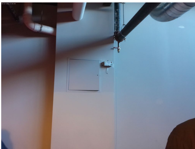
7. 12/19/22 – View of SSDS #3 Manometer Enclosure
