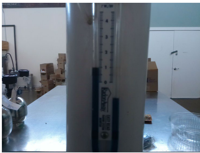
9. 12/19/22 - View of SSDS #4 Manometer Reading
