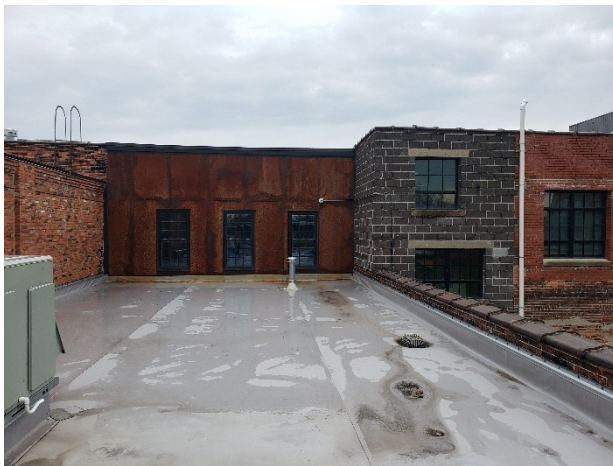
21. 1/13/25 – View of roof top enclosure for SSDS-5 blower.
