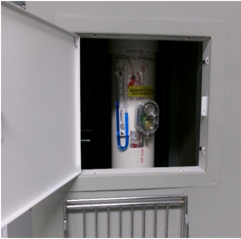
17. 1/13/25 – View of SSDS-1 and alarm located inside of the ODL suite.
