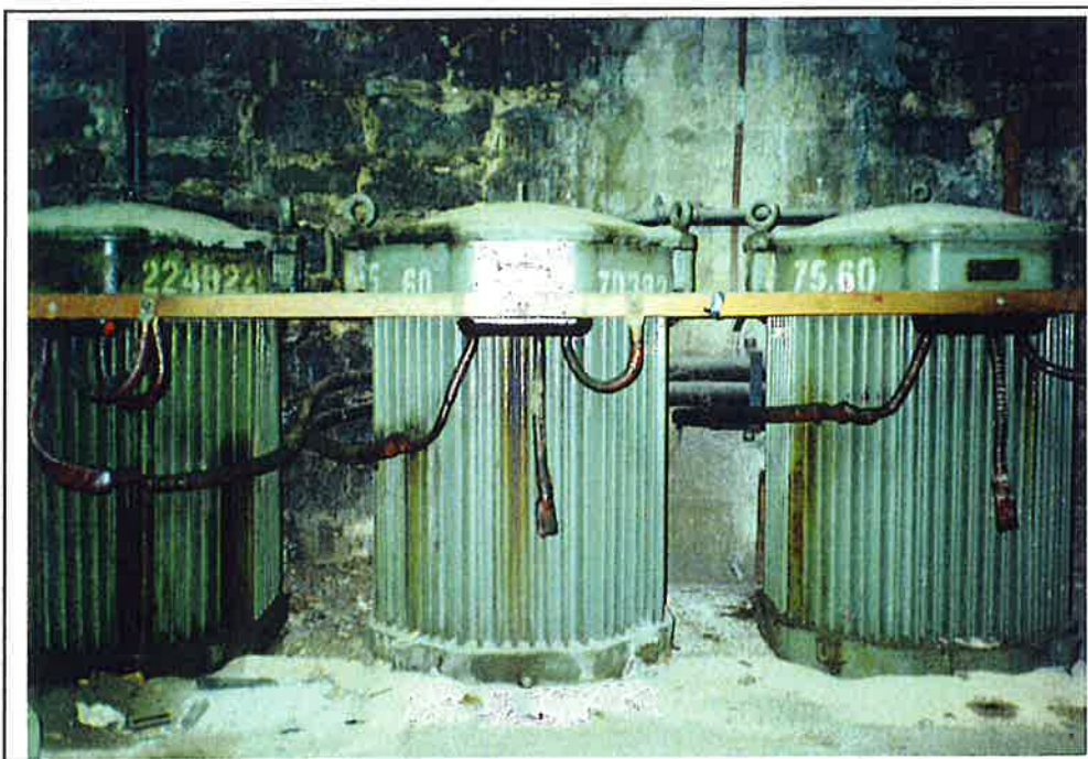
Basement, 75 kVA transformers
