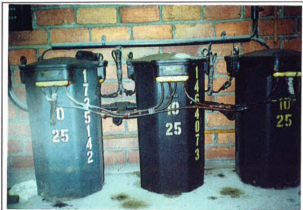
Basement, 10 kVA transformers
